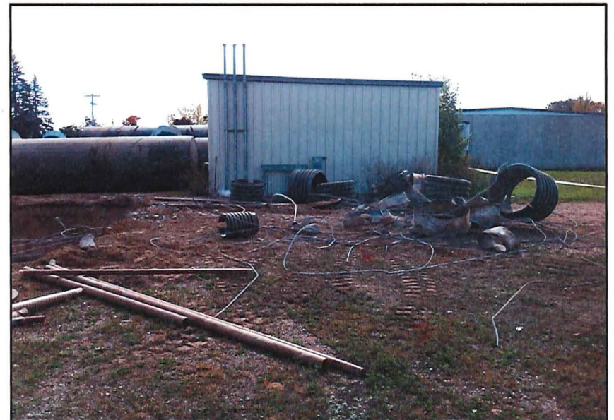
Facing South - Vent Pipes Attached To Parking Garage
