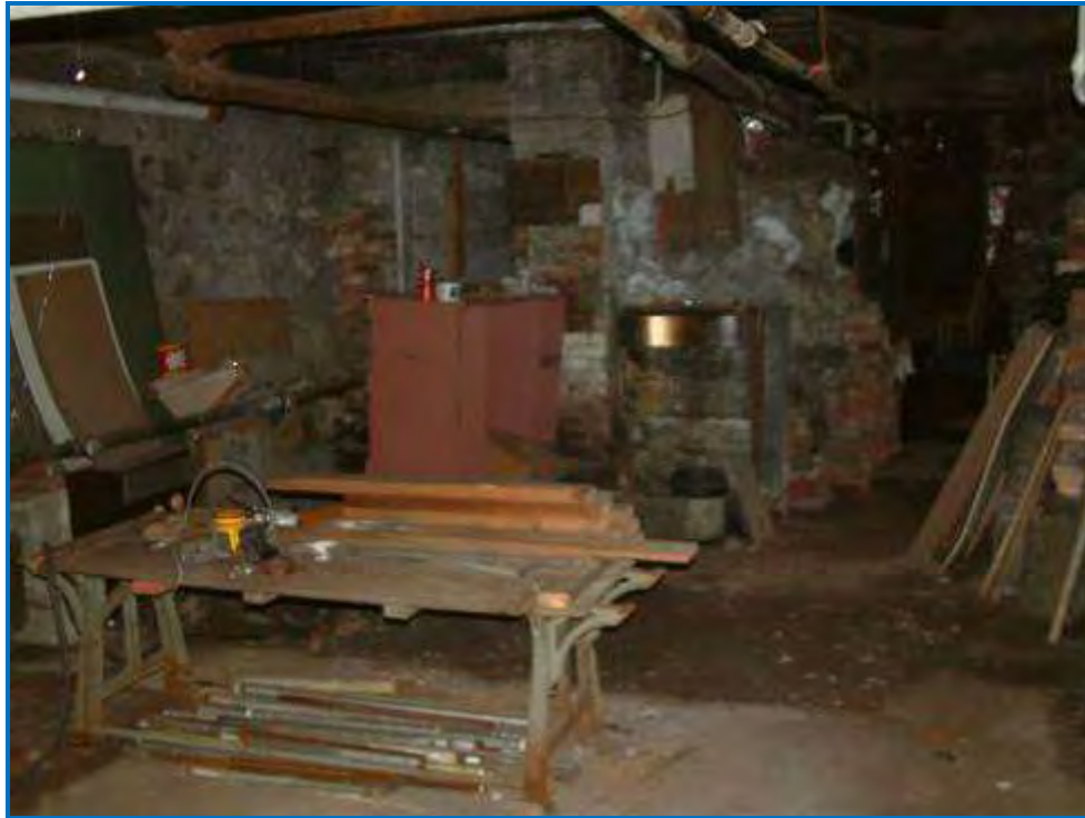
Photo #9 Basement. Structure is old, dingy, and wet, but solid. No rats.
