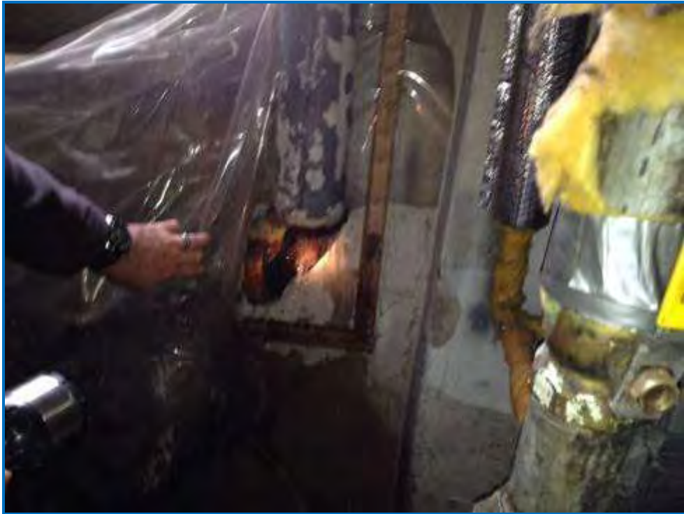
Photo #31 Roof drain plumbing in the dry cleaning room is severed, and all rain comes directly into the building, washing whatever is on the floor into the drain.
