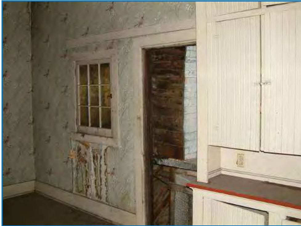
Photo #51 Second floor, kitchen. Water damage is everywhere.
