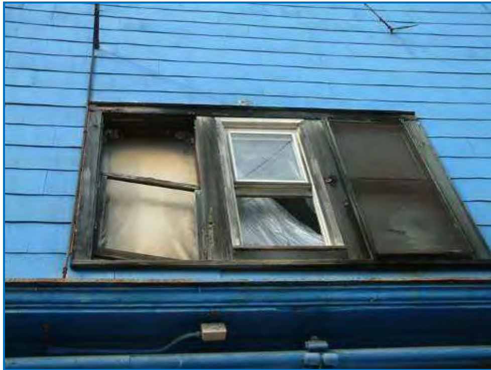
Photo #3 Second floor apartment on the Property . Windows are completely gone.
