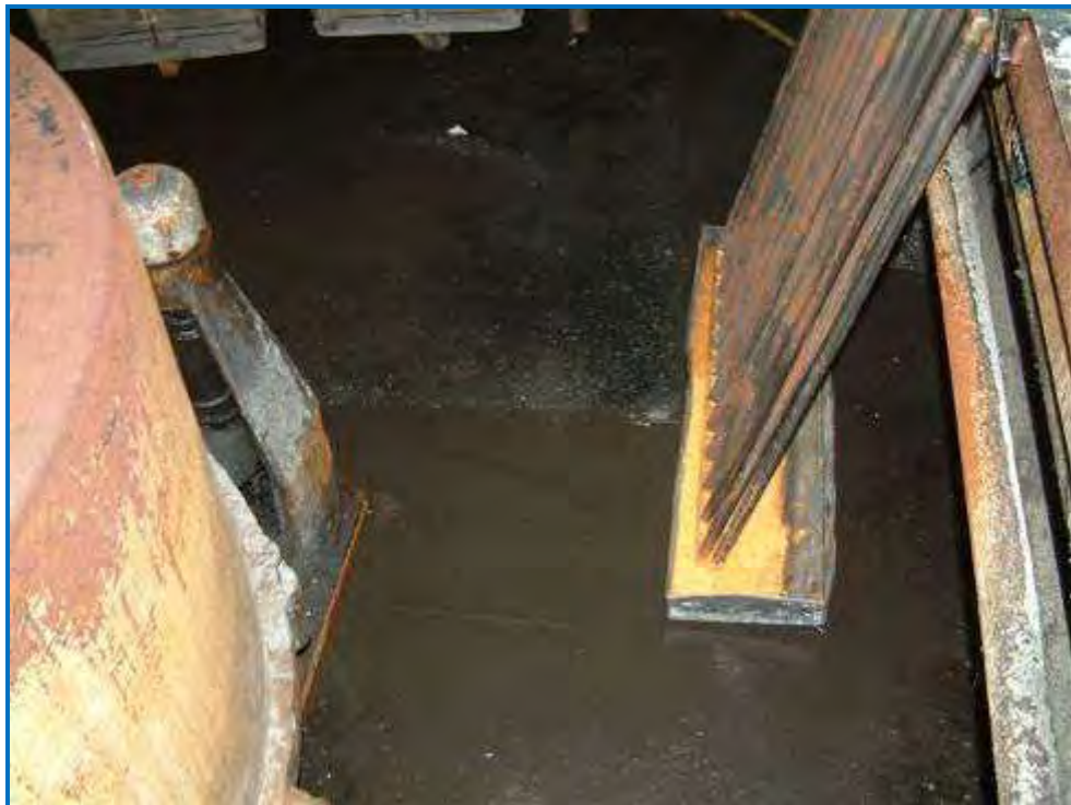
Photo #26 The entire dry cleaning area floods when it rains from leaks in the roof, walls, and windows.
