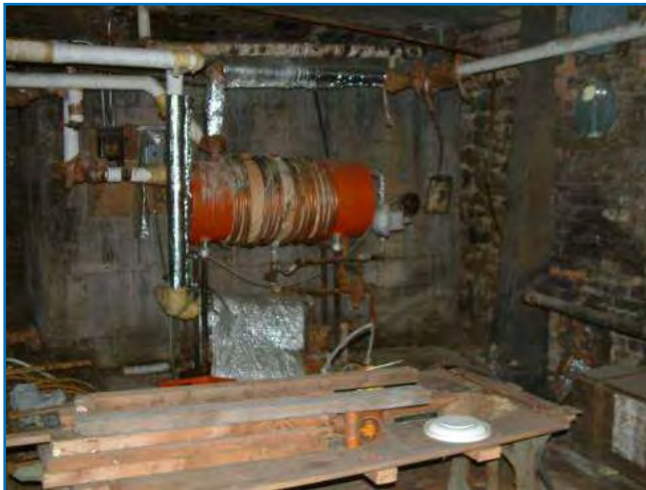
Photo #14 Basement, the solvent condenser/distillation unit. The sanitary sewer pipe is higher than the solvent condenser/distillation unit; therefore, there is no obvious place to discharge solvent-contaminated water to the sewer. A small pit (not visible here, see Photo #15) is adjacent and on the right side of the distillation unit.
