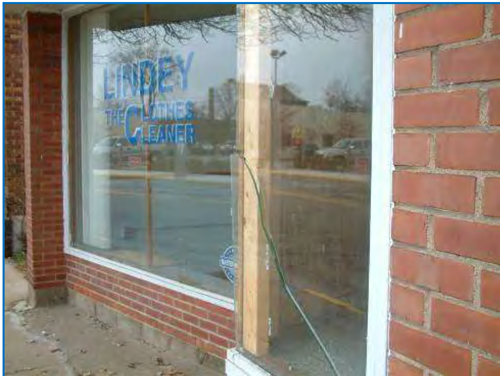
Photo #6 Broken glass is noted in the storefront and could pose a safety hazard or point of illegal entry.
