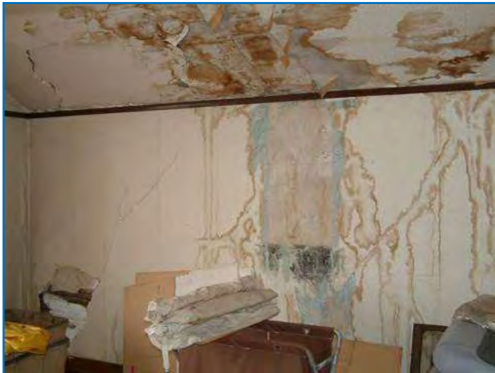
Photo #52 Second floor apartment. Water damage looks like this throughout the second floor, and indicates failure of the second floor structure is in progress.
