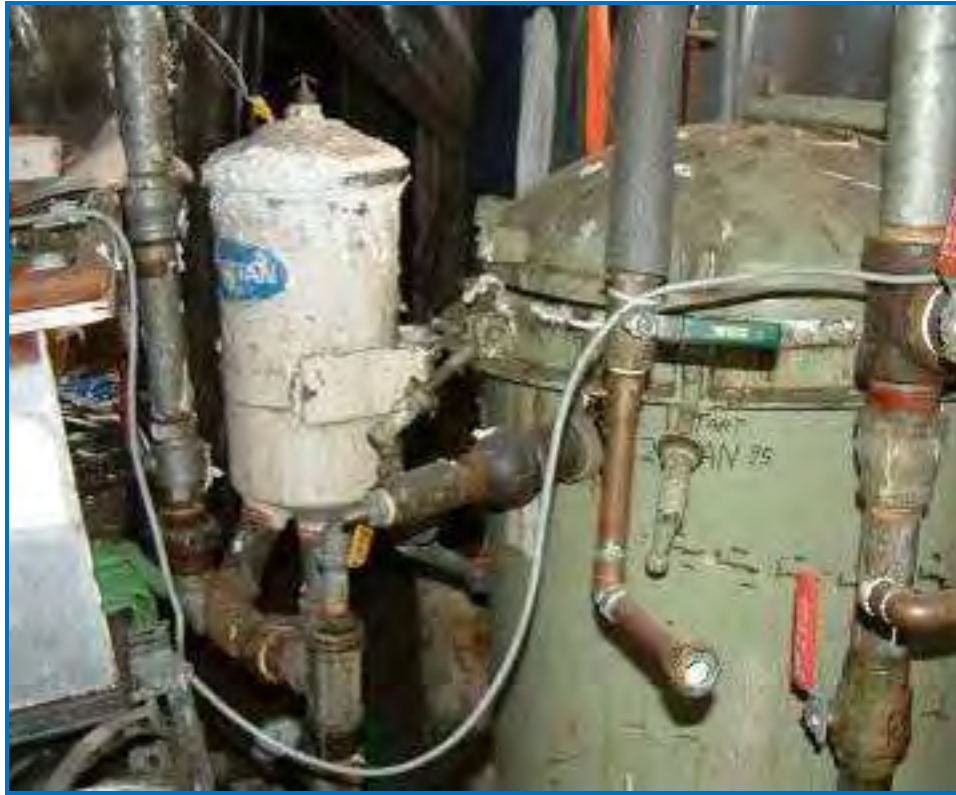
Photo #37 Lint and button filter in the dry cleaning cycle. Filter materials are hazardous waste.
