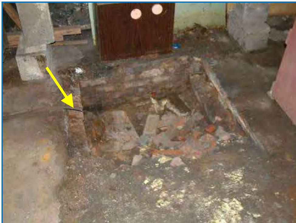
Photo #15 Small pit in the basement cited as a REC. This sump is adjacent to the solvent distillation unit shown in Photo #14, and could have been used to discharge solvent/water mixtures. Note the black hose discharging to the sump on the left.
