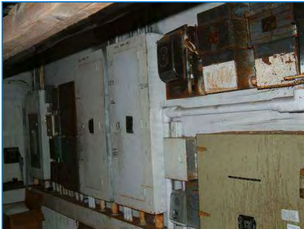
Photo #48 Electrical panel in the hall between the steam laundry and the dry cleaning room.
