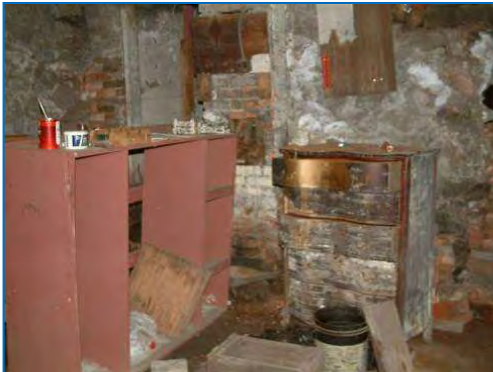
Photo #10 Basement. Evidence of water damage.
