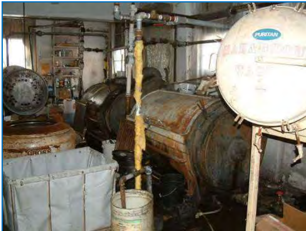
Photo #22 Looking southwest. General view of recent dry cleaning area. The two large older dry cleaning machines on the right have solvent in them.
