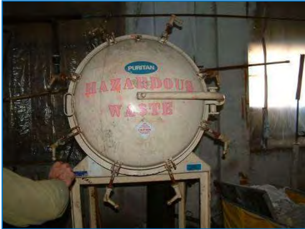
Photo #21 Dry cleaning equipment room, solvent filter.
