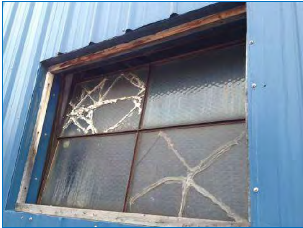
Photo #7 Back of the building. Open windows are allowing rain to pour in, and could be an entry point for illegal access.
