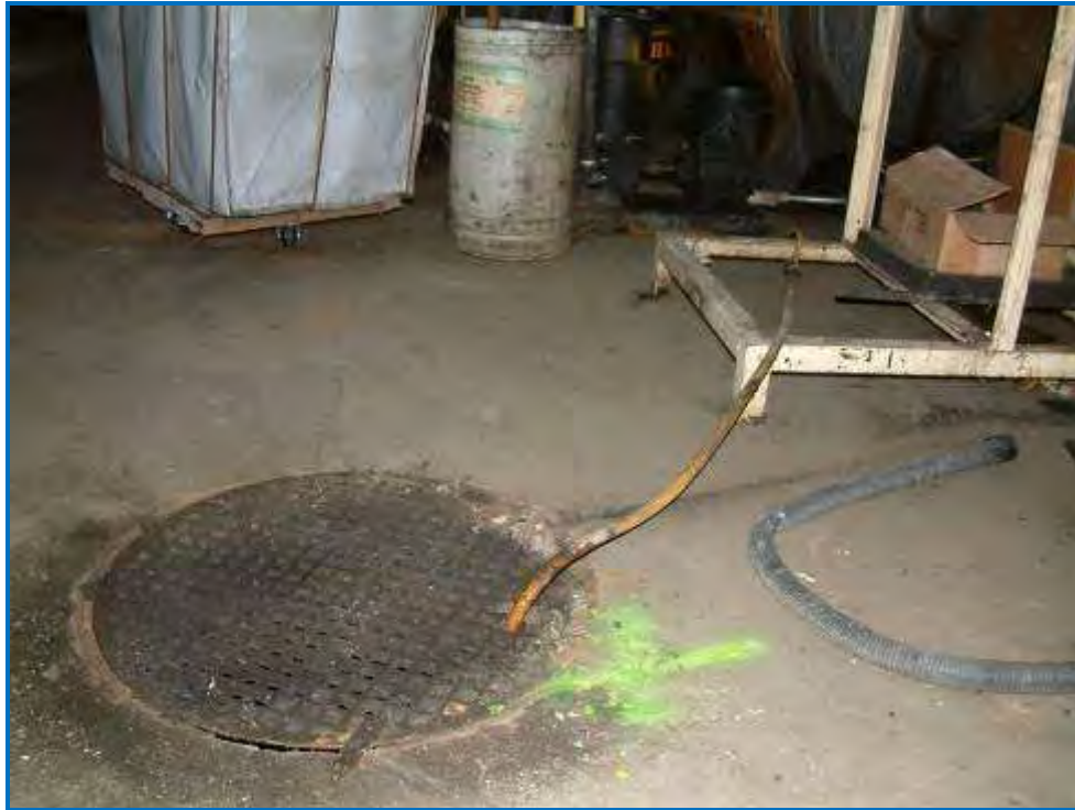
Photo #27 Old brick sanitary sewer (36-inch) in modern dry cleaning room. This brick sewer leaks, as evidenced during rain storms and dropping water levels. Notice the yellow hose draining into the sewer (see Photo 28 for more).
