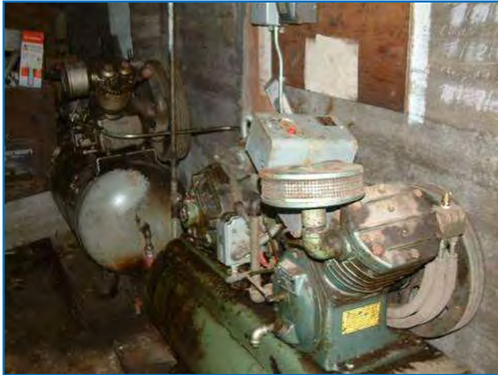
Photo #13 Twin compressors in the basement near the stairs.
