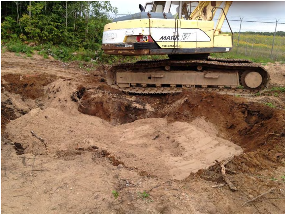
Photo #12 Backfilling the primary spill area with sand recovered from the well development activities.
