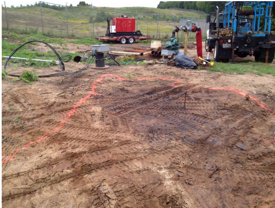
Photo #2 Primary Spill Area, looking northeast toward the Airport Fence. The new City Well is in the background.
