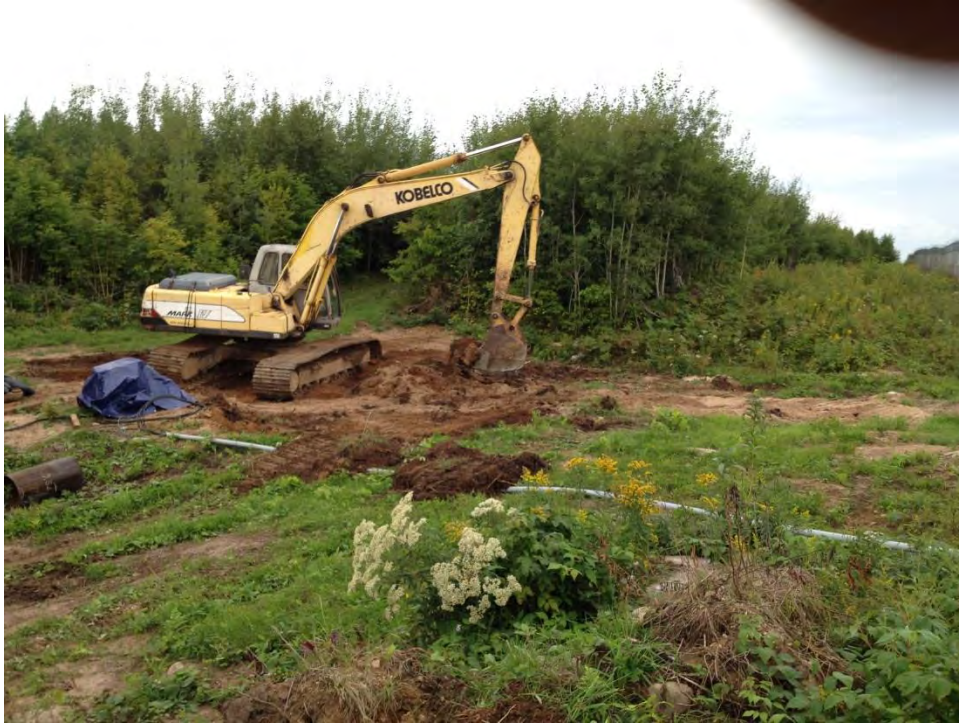
Photo #13 Backfilling of both primary and secondary areas is complete at 4:40 PM, September 3, 2014.
