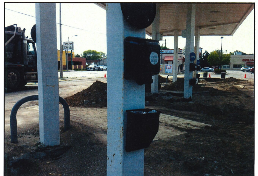
Dispenser Island - Piping Sampling
