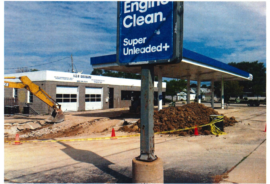
Tank Bed - South of Pump Island
