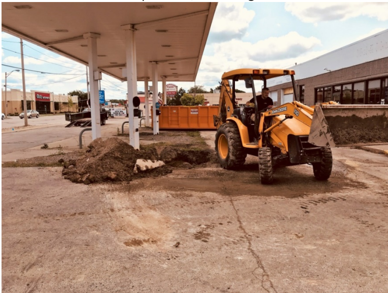
Clean-up and loading of contaminated soil to be transported to Waste Management Bristol, WI. Bio-pile
