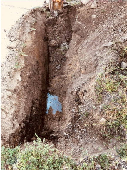
Initial excavation trench following former pipeline south of SS14. No sheen observed on perched, shallow groundwater.
