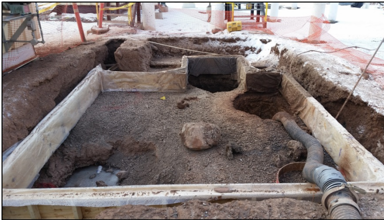
Photo 2: The Line 1 excavation with concrete foundation form. The contaminated soil was located in the bottom left corner. Photo facing southwest on November 21, 2014.
