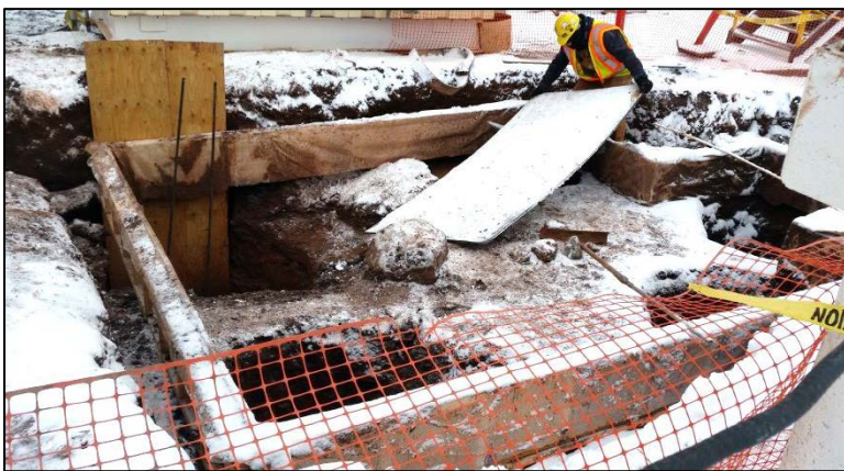
Photo 3: The Line 1 excavation with foundation form and Sonotube borings. The contaminated soil was located in the upper left corner. Photo facing south on November 24, 2014.
