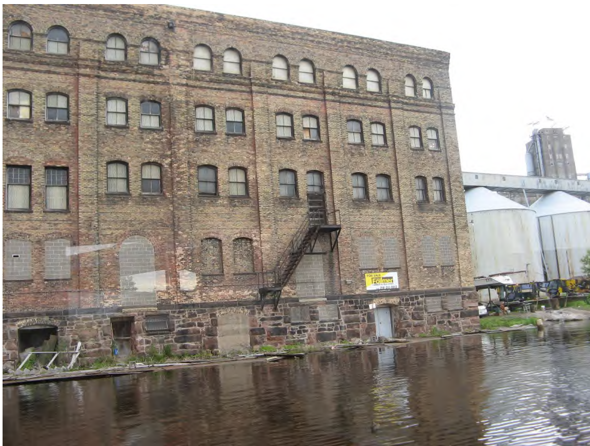
Warehouse for sale in Hughitt Slip—cracks in bricks & mortar were evident from top to bottom at right corner.
