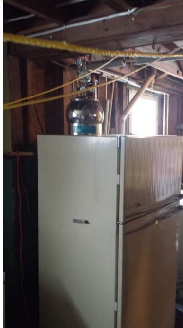
Photo 5: 720 East 5 th Street – Indoor air sample. February 22, 2016.
