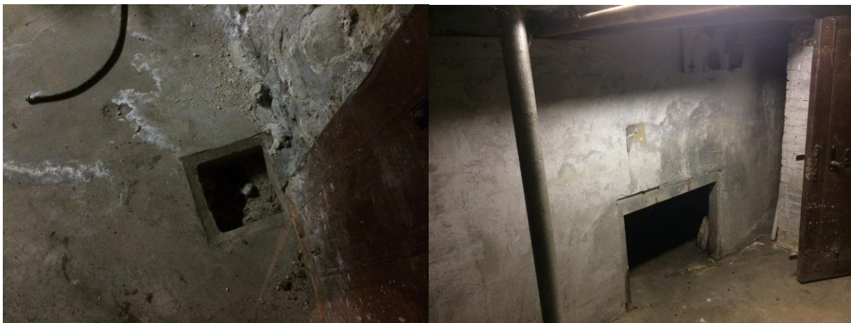
Picture 7 – left: Square void space in concrete floor in the southeast corner of boiler room
