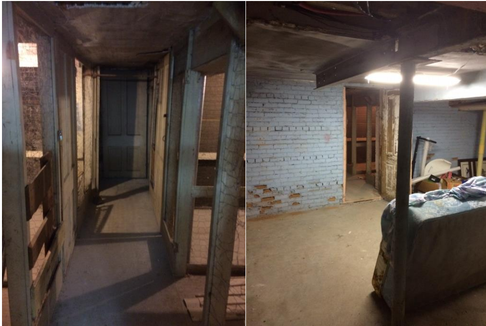
Picture 1 – left: Looking south at southernmost storage room, individual storage unit setup. Picture 2 – right: Looking south-southwest at doorway to individual storage unit room and next storage room to the north.
