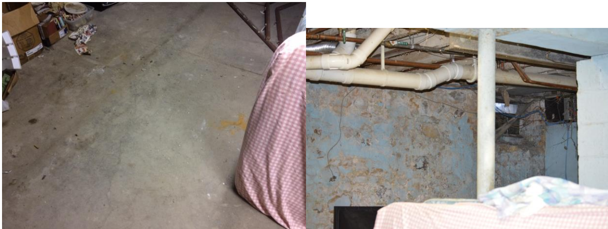
Picture 3 – left: Typical concrete floor condition – minimal cracks Picture 4 – right: Looking at west wall and window well.
