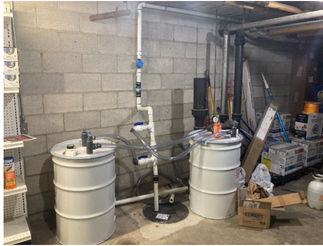
IMAGE OF SUMP 2 AND ASSOCIATED REMEDIATION SYSTEM; PVC PIPING CONNECTS TO DISCHARGE LINE THAT RUNS THROUGH SOUTHERN WALL OF ACE HARDWARE BASEMENT (OUTFALL 011)
