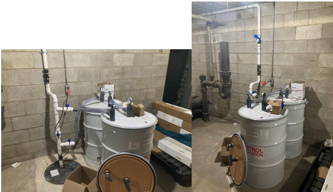
IMAGE OF SUMP 3 AND ASSOCIATED REMEDIATION SYSTEM; PVC PIPING CONNECTS TO DISCHARGE LINE THAT RUNS THROUGH SOUTHERN WALL OF ACE HARDWARE BASEMENT (OUTFALL 011)
