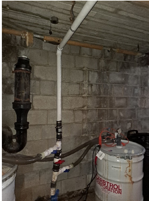
IMAGE OF SUMP 1 AND ASSOCIATED REMEDIATION SYSTEM; PVC PIPING CONNECTS TO SUMP 3 PIPING THAT RUNS TO DISCHARGE THROUGH SOUTHERN WALL OF ACE HARDWARE BASEMENT (OUTFALL 011); SUMP 1 NO LONGER DISCHARGES TO OUTFALL 001 (OUT-OF-SERVICE)
