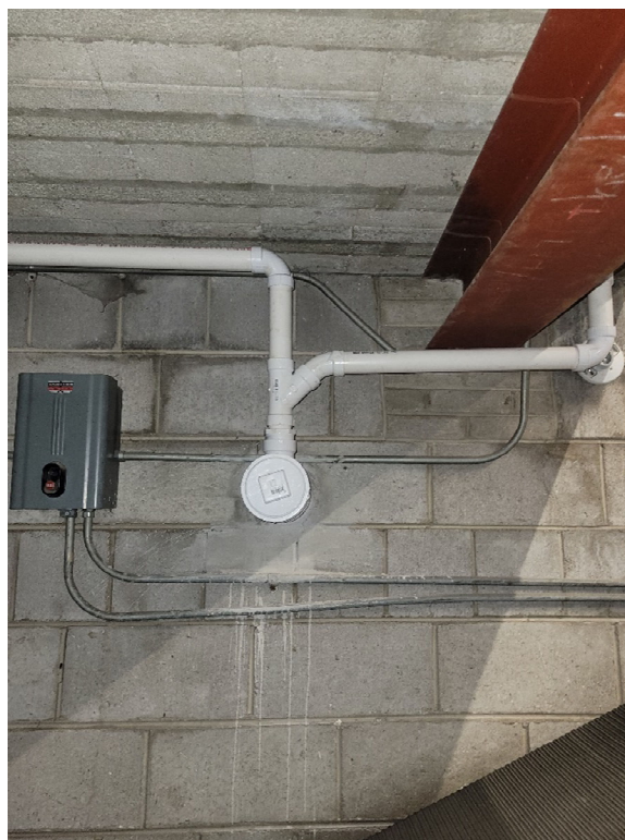
IMAGE OF DISCHARGE LINE THAT RUNS THROUGH SOUTHERN WALL OF ACE HARDWARE BASEMENT (OUTFALL 011); SAMPLE PORT IN BOTTOM OF DISCHARGE LINE NOT PICTURED
