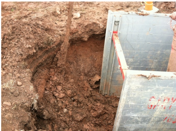
Photo 3: Fire hydrant replacement excavation on 11/7/2012. Soil with discoloration and a petroleum odor is visible on left side of the photo approximately three feet below ground surface.
