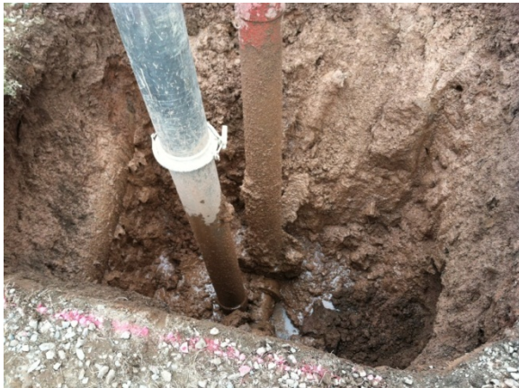
Photo 2: Fire hydrant replacement excavation on 11/1/2012. Sheen was observed on the water and on the wet soil in the bottom of the excavation. The dark gray pipe is the hydrovac truck hose and the red pipe is the fire hydrant.
