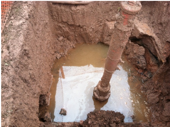
Photo 5: Office water valve excavation. A sheen was observed on the water surface and on wet soil. The pipe in the photo is the water valve that was being replaced.
