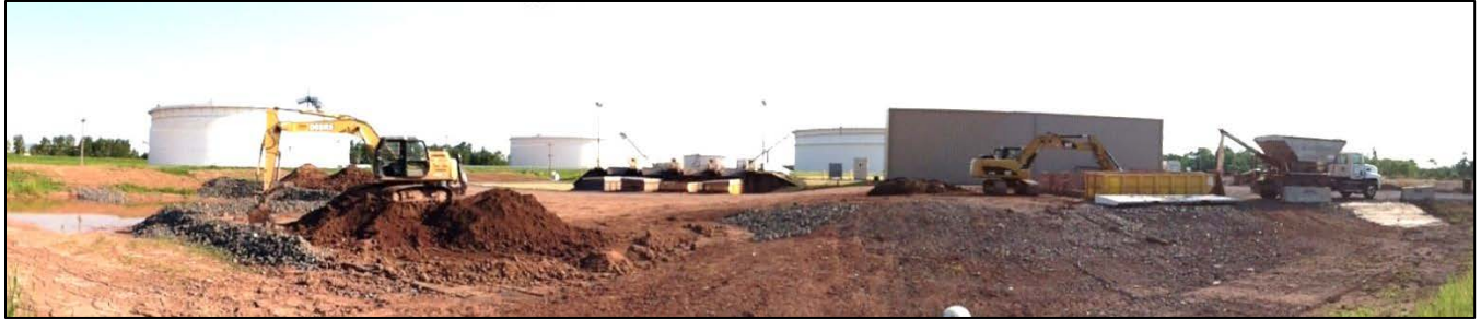
Photo 4: The permanent SMA Facility unimpacted slurry soil stockpile area. The unimpacted slurry soil solidification roll-off containers are on the right side of the photo; the unimpacted solidified slurry soil stockpiles are on the left. The photo was taken facing northeast on August 12, 2013.
