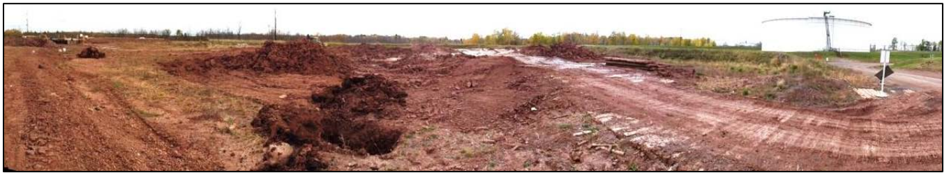
Photo 1: The SMA prior to permanent Facility construction. The photo was taken facing southwest on October 9, 2012.
