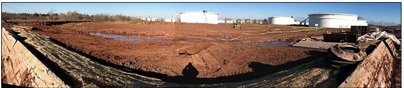
Photo 2: The SMA prior to permanent Facility construction. The photo was taken facing northwest on November 13, 2012.
