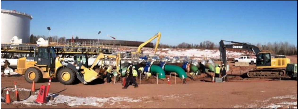
Photo 1: Manifold 225 release area with remedial response personnel and equipment. Photo taken facing north on December 3, 2014.
