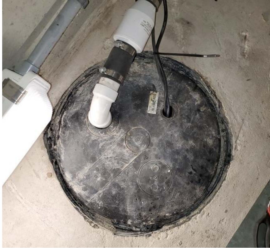
Photograph 3: Sump lid with openings for cord and piping
