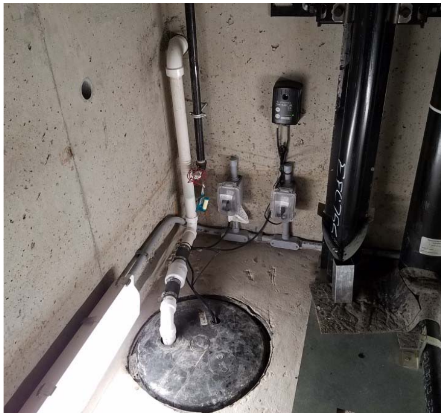
Photograph 2: Sump and discharge piping
