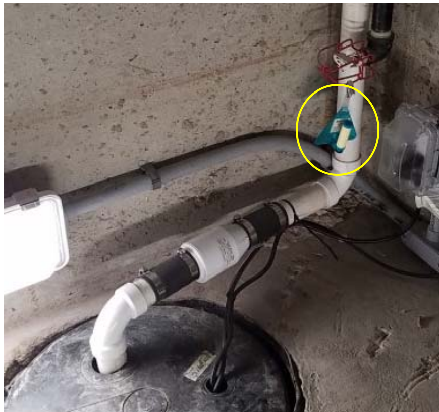
Photograph 4: radiello passive air sampling device deployed above sump
