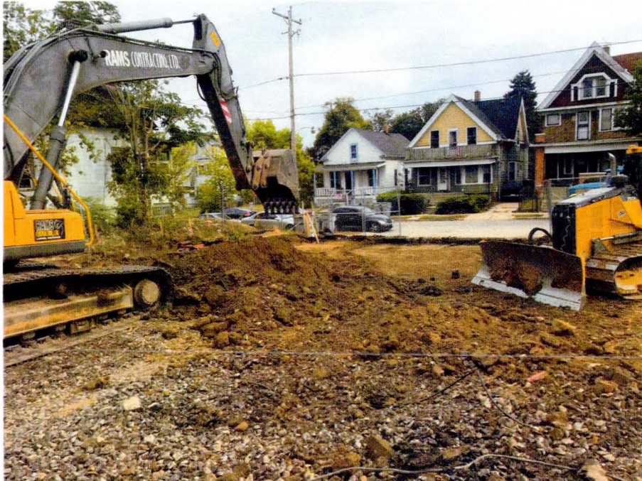
Photo 1: Parking lot subgrade removal in progress in northeast portion of Site on October 2, 2017. View looking to northeast.
