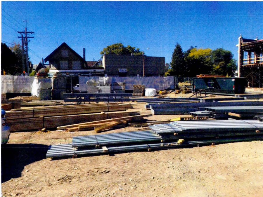
Photo 8: First 18 inches of clay placed for green space soil cover system in south portion of Site (currently used for outdoor staging) on October 4, 2017. View looking to west.
