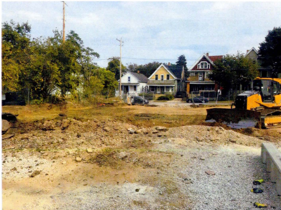
Photo 2: Parking lot subgrade removal in progress in northeast portion of Site on October 2, 2017. View looking to east.
