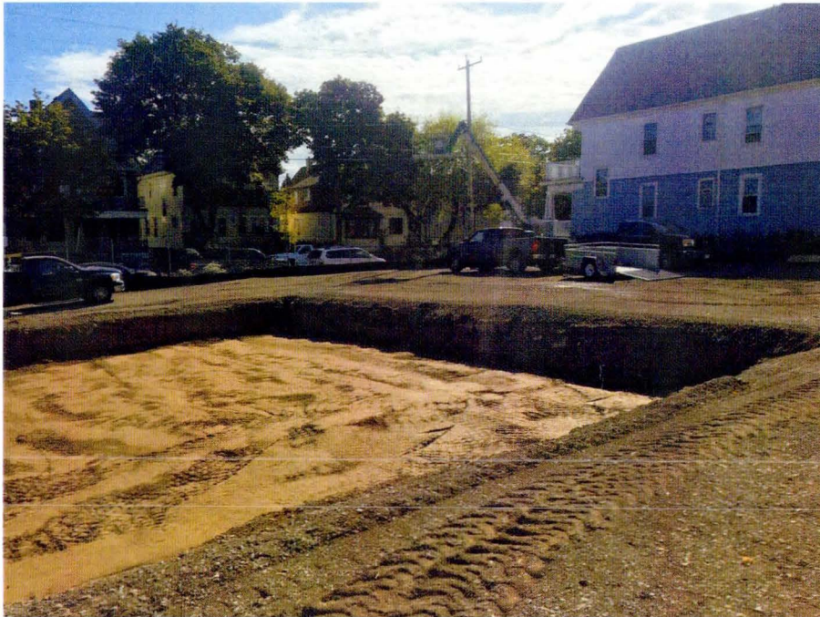
Photo 7: Gravel subgrade placed and compacted in northeast portion of Site for new asphalt parking lot on October 4, 2017. View looking to southeast.
