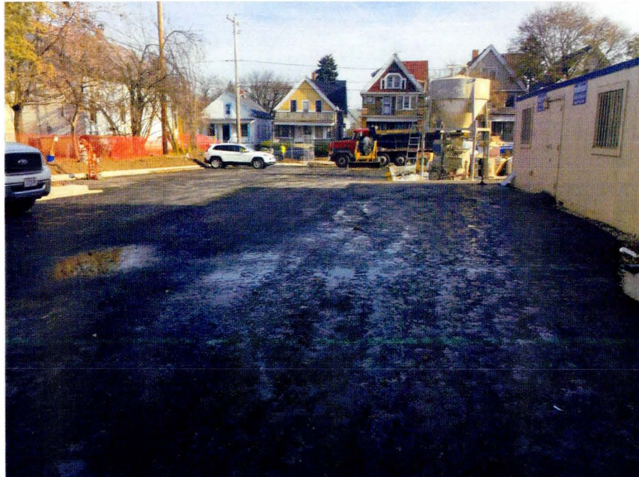
Photo 10: Asphalt binder course installed in north and northeast portion of Site on November 13, 2017. View looking to east.
