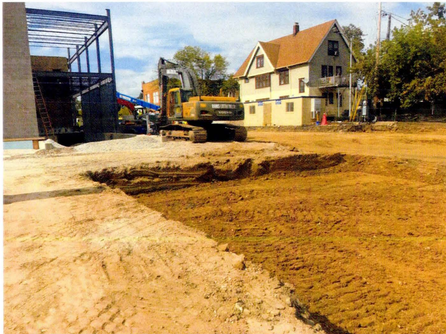
Photo 4: Parking lot subgrade removal (including area for pervious pavers and underlying storm water retention) in north-northeast portion of Site on October 3, 2017. View looking to northwest.
