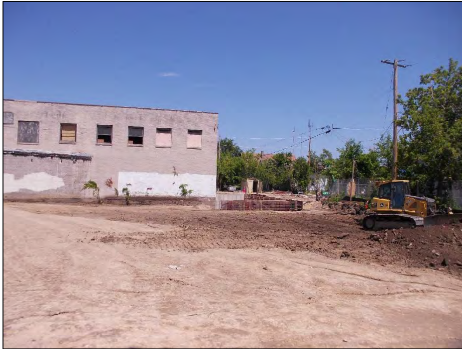
Photo 7: Grading and subgrade preparation activities in south green space area on July 19, 2017. View looking north.
