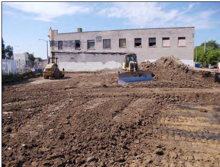
Photo 6: Excavation, grading, and subgrade preparation activities in south green space area on July 18, 2017. View looking north-northwest.
