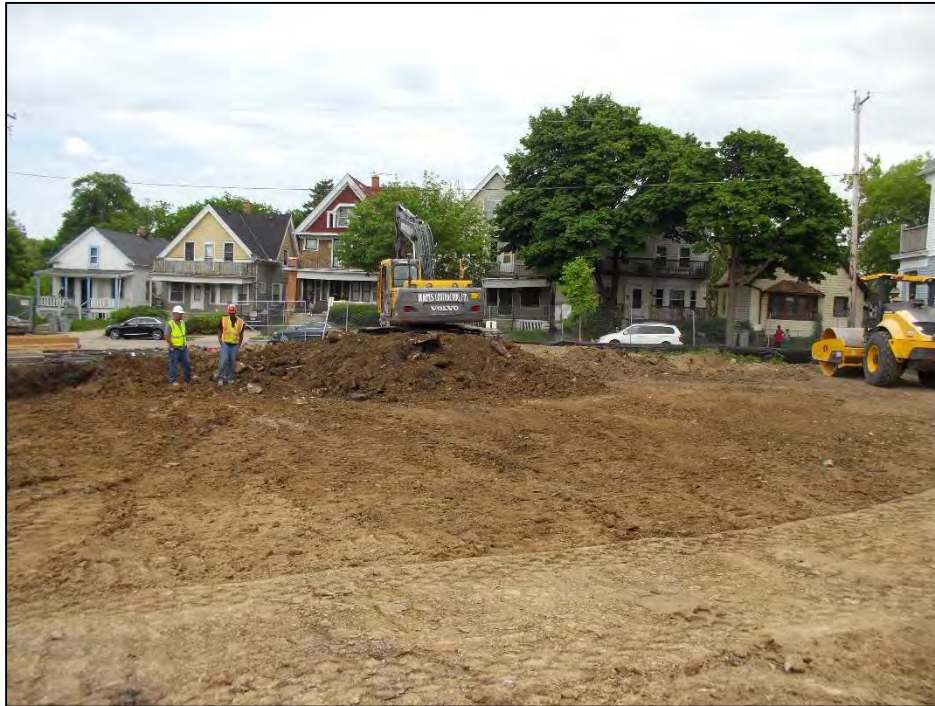
Photo 3: Excavation in new east parking lot area on June 8, 2017. View looking east.
