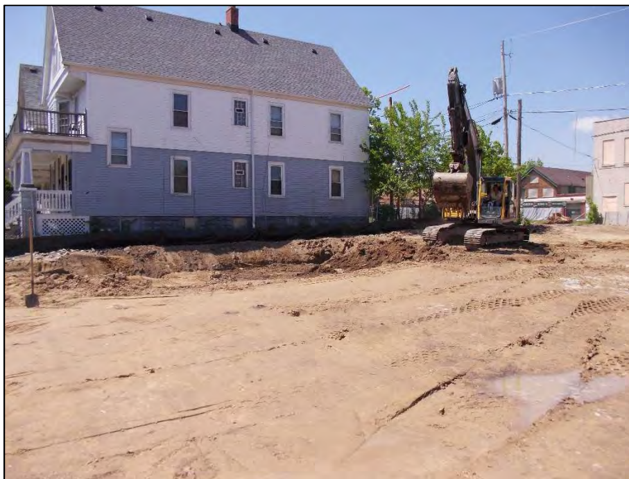
Photo 4: Excavation, backfilling, and grading activities in new east parking lot area on June 9, 2017. View looking southwest.
