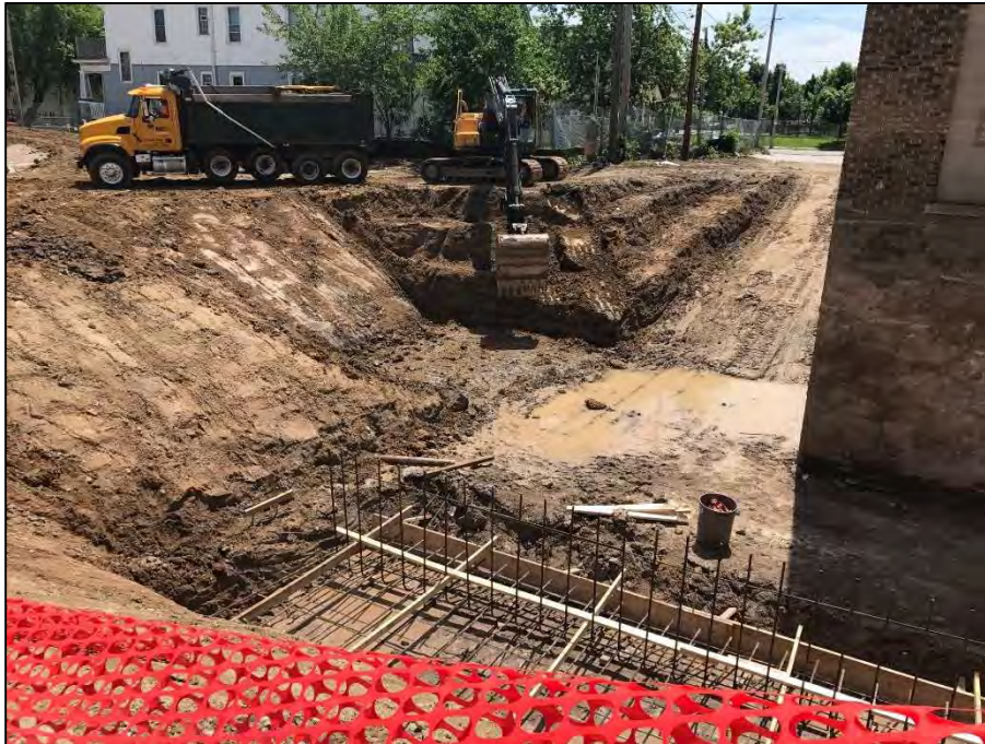
Photo 5: Excavation in eastern portion of new basement area on June 14, 2017. View looking southeast.
