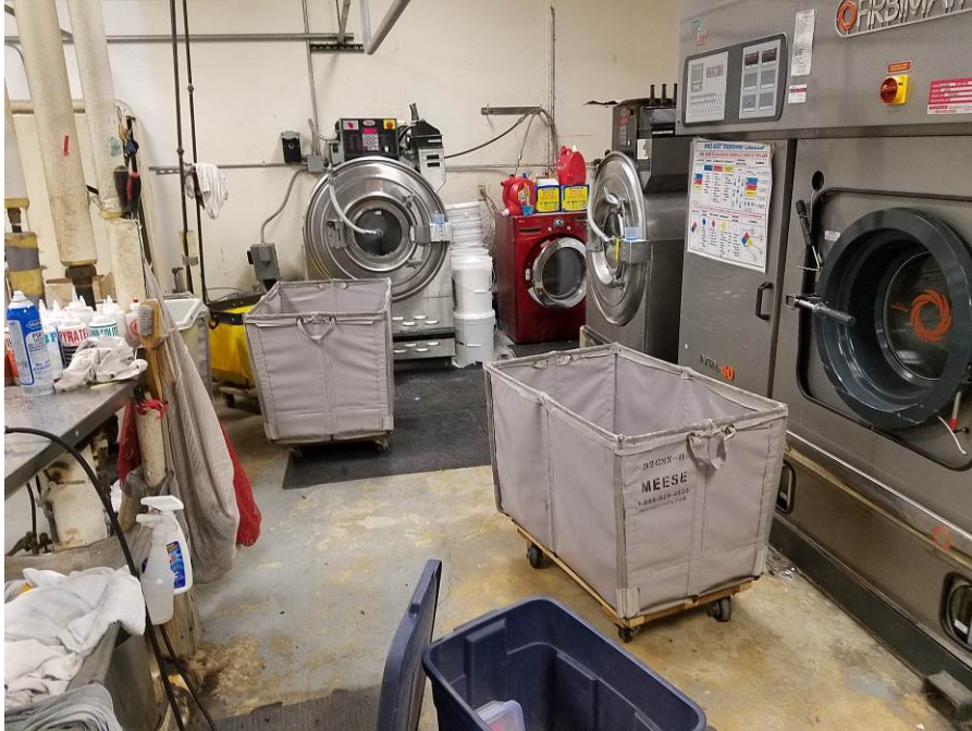
Photo 3: Looking west at dry cleaning machines inside dry cleaner unit (January 19, 2017).
