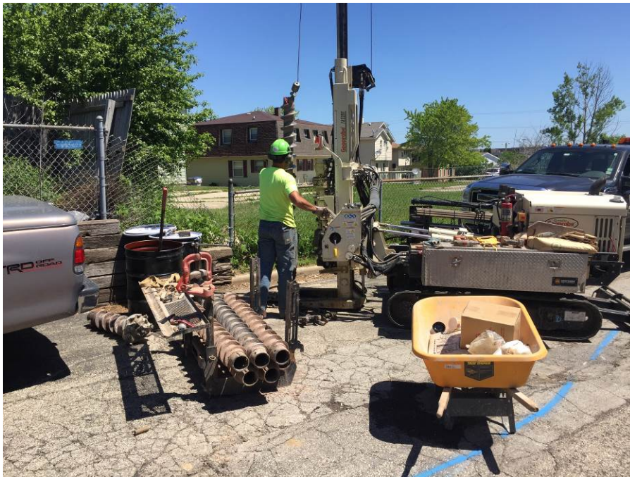
Photo 6: Looking northeast at monitoring well MW-3 installation from alleyway behind dry cleaner unit (June 1, 2017).
