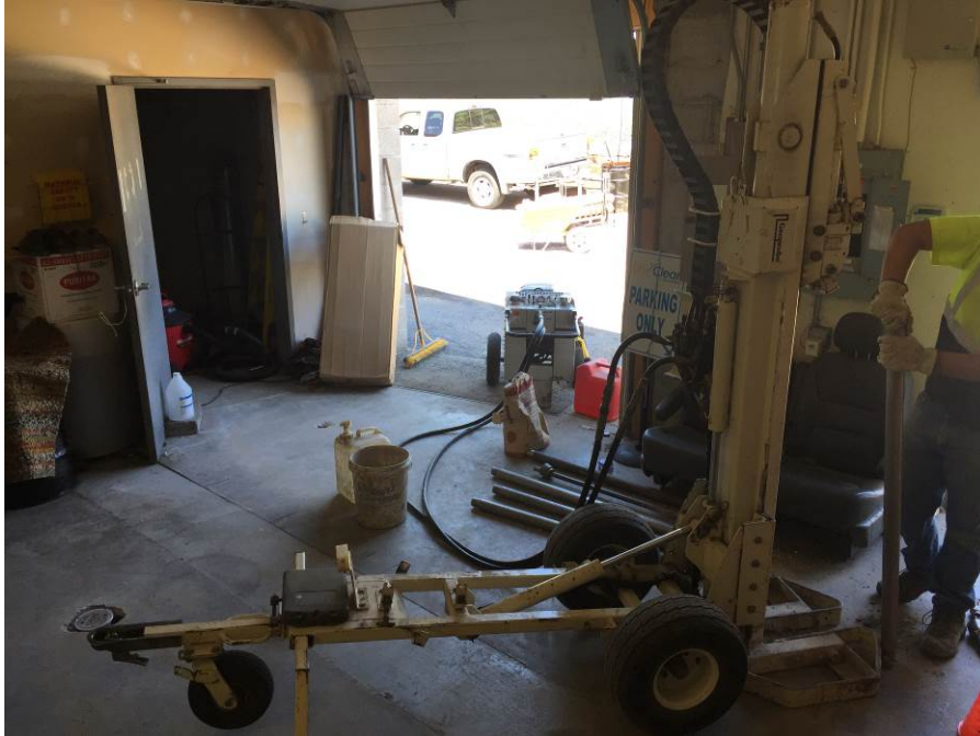
Photo 5: Looking northwest inside north end of dry cleaner unit during installation of boring GB-5 (June 1, 2017). Boring GB-4 is visible in the floor in front of the utility room doorway. Monitoring well MW-3 (prior to surface sealing) is visible in the floor on the left side of the photo.
