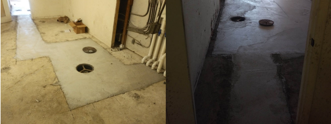
VIEWS OF CONCRETE PAVEMENT FLOOR SLAB OF 2410 TENANT SPACE AFTER CHEMICAL TREATMENT AND SUB-SLAB DEPRESSURIZATION SYSTEM INSTALLATION/PRIOR TO OCCUPANCY BY TENANT; CONCRETE PAVEMENT IMPLEMENTED AS ENGINEERED BARRIER
