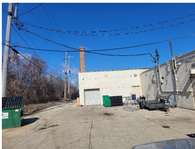
VIEW OF ASPHALT PAVEMENT WITHIN WESTERN (REAR) DRIVEWAY BEHIND 2410 & 2412 TENANT SPACES IMPLEMENTED AS ENGINEERED BARRIER
