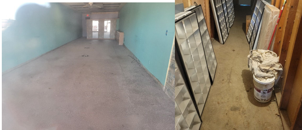
VIEW OF CONCRETE PAVEMENT FLOOR SLAB OF 2412 TENANT SPACE AFTER CHEMICAL TREATMENT AND SUB-SLAB DEPRESSURIZATION SYSTEM INSTALLATION/PRIOR TO OCCUPANCY BY TENANT; CONCRETE PAVEMENT IMPLEMENTED AS ENGINEERED BARRIER
