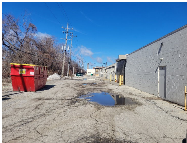
VIEW OF ASPHALT PAVEMENT WITHIN WESTERN (REAR) DRIVEWAY BEHIND 2414 & 2414B TENANT SPACES IMPLEMENTED AS ENGINEERED BARRIER
