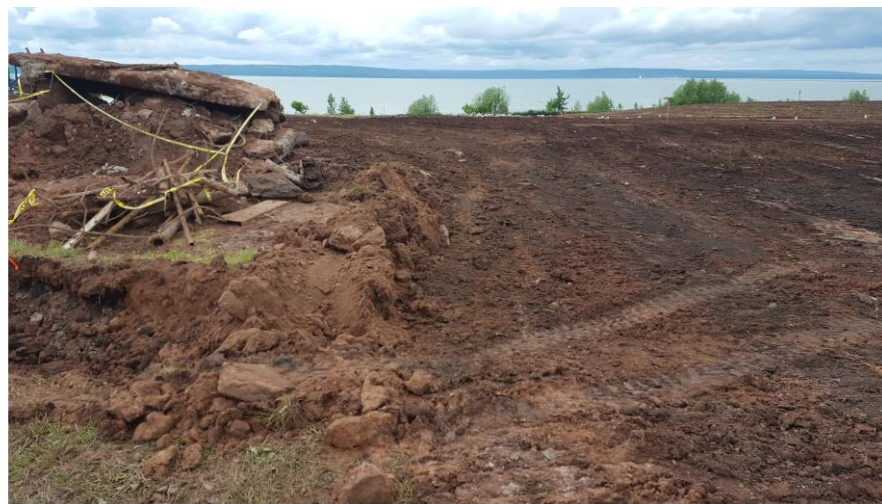
Location of excavation of petroleum impacted material and debris pile looking north.
