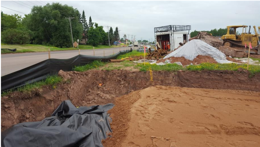
Location of unknown petroleum product after excavation looking west.
