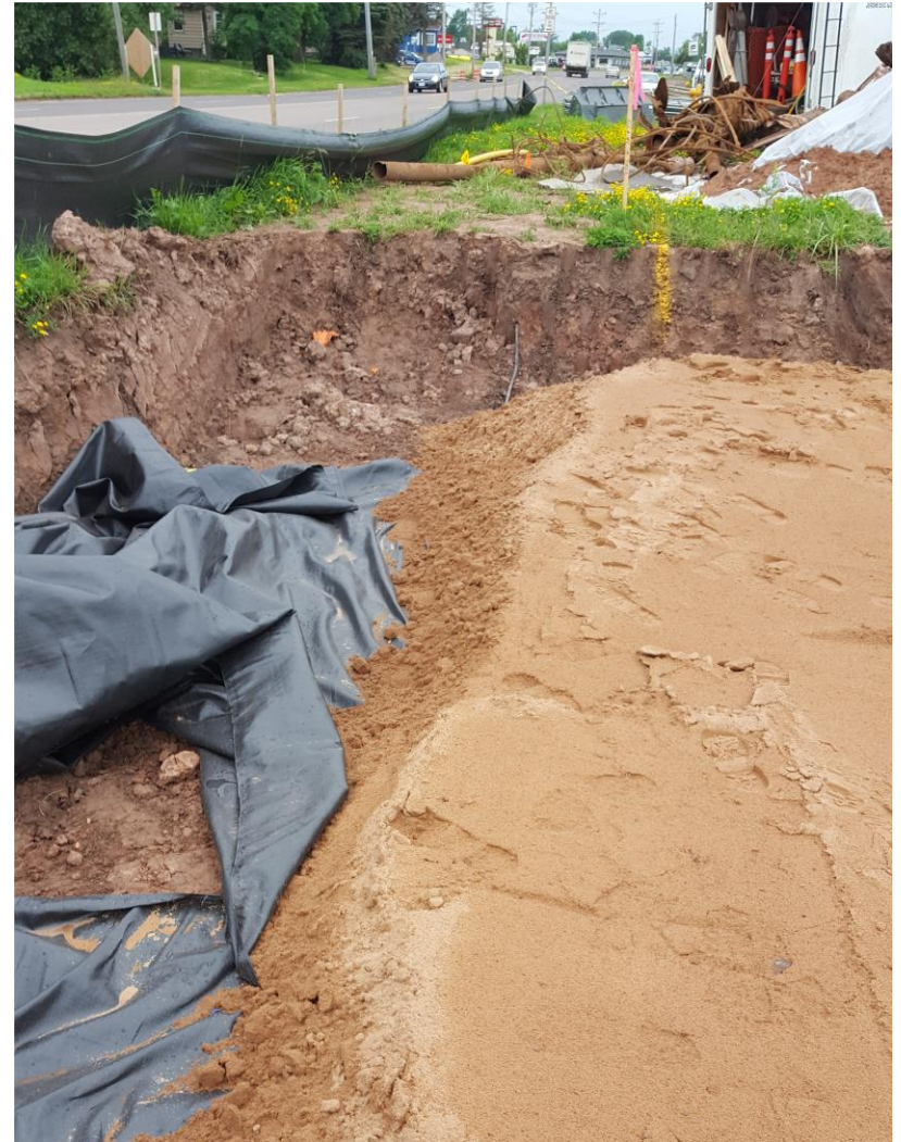
Location of unknown petroleum product after excavation looking west.
