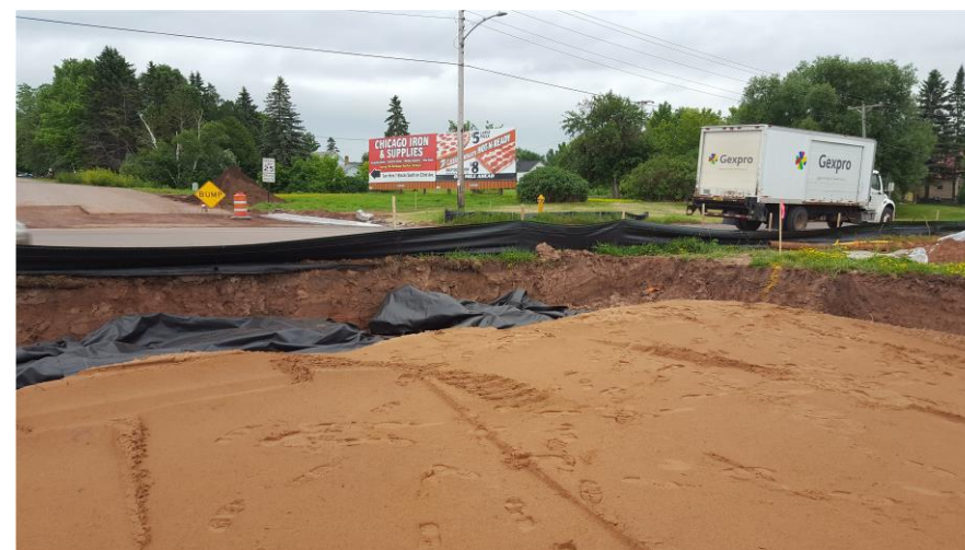
Location of unknown petroleum product after excavation looking south.
