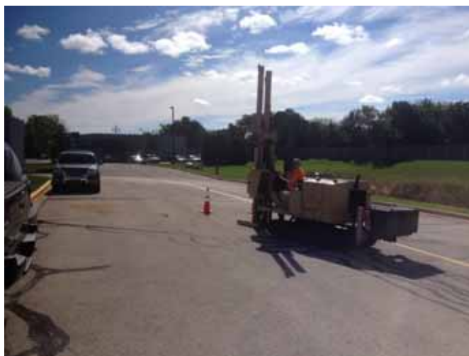
Photo No. 3 showing the advancement of a boring (TW-1) in the driveway south of the Bright Cleaners tenant space, view to the east.
