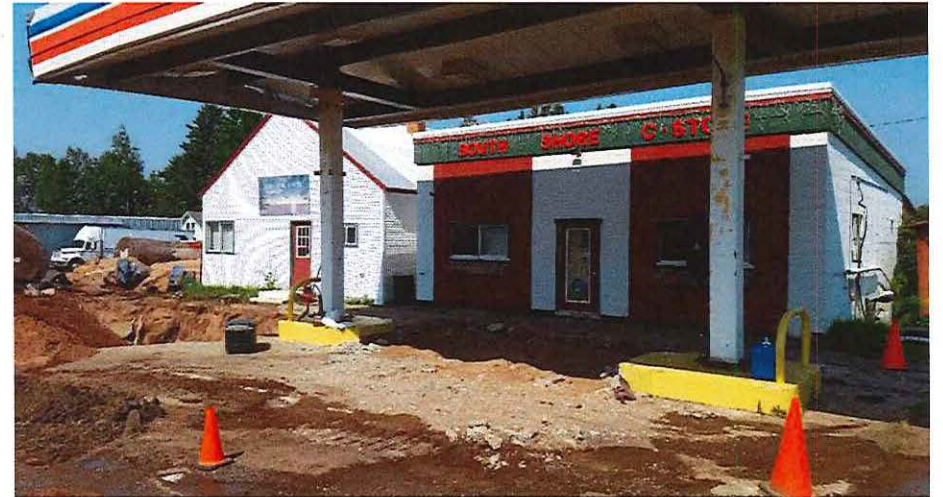
View of C-Store buildings and dispensers facing northwest.
