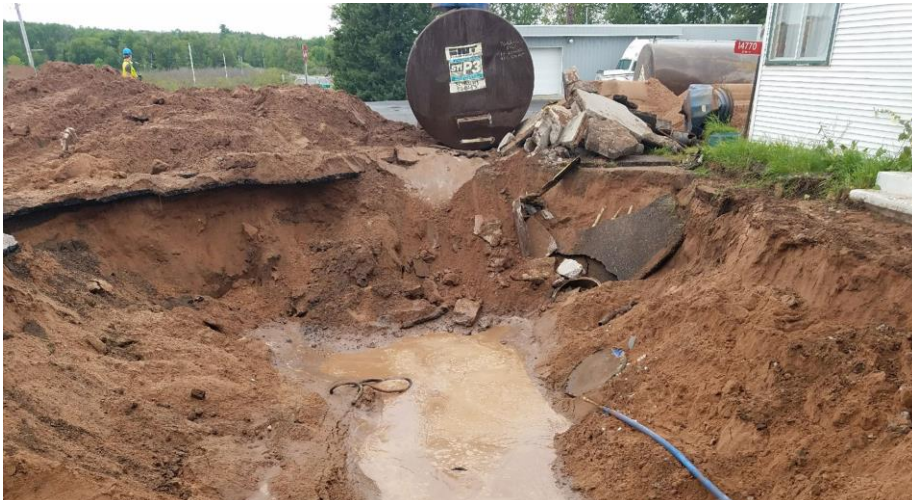
View of groundwater filling excavation.
