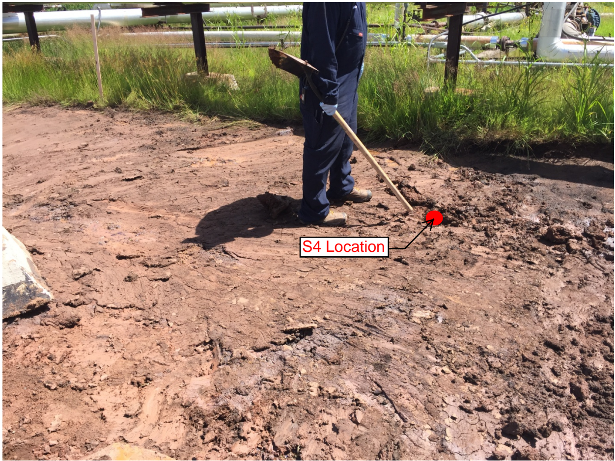
Photo 12: Looking south at the sample location S4 after the final round of excavation.
