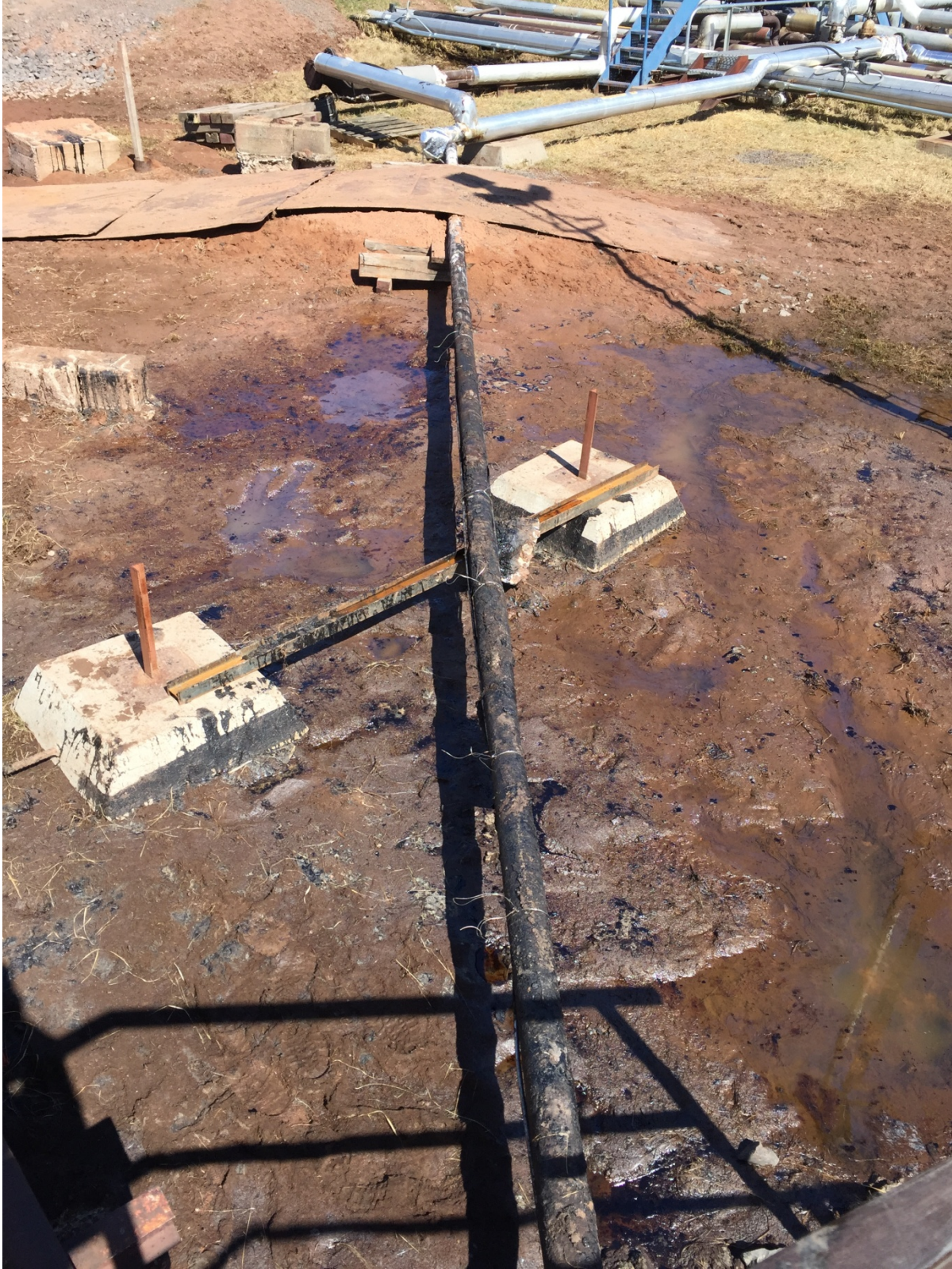
Photo 6: Looking northeast at the site after first round of excavation. The pipes insulation had been removed and some product can be seen seeping into the excavation. This was removed in subsequent excavations.
