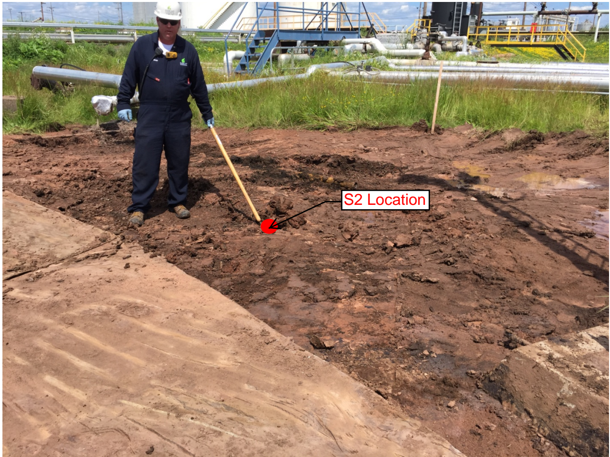
Photo 10: Looking northeast at the sample location S2 after the final round of excavation.
