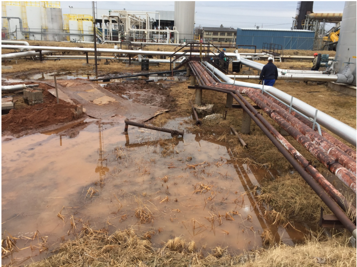
Photo 8: Looking south at the release site. Please note the sand dam which functions to isolate any water that accumulates in the excavation from the stormwater in the rest of the tank dike bottom. There are also a number of abandoned pipes in the area that hindered excavation in some places. Laborers can be seen conducting hand excavation of contaminated soil underneath the pipe rack.
