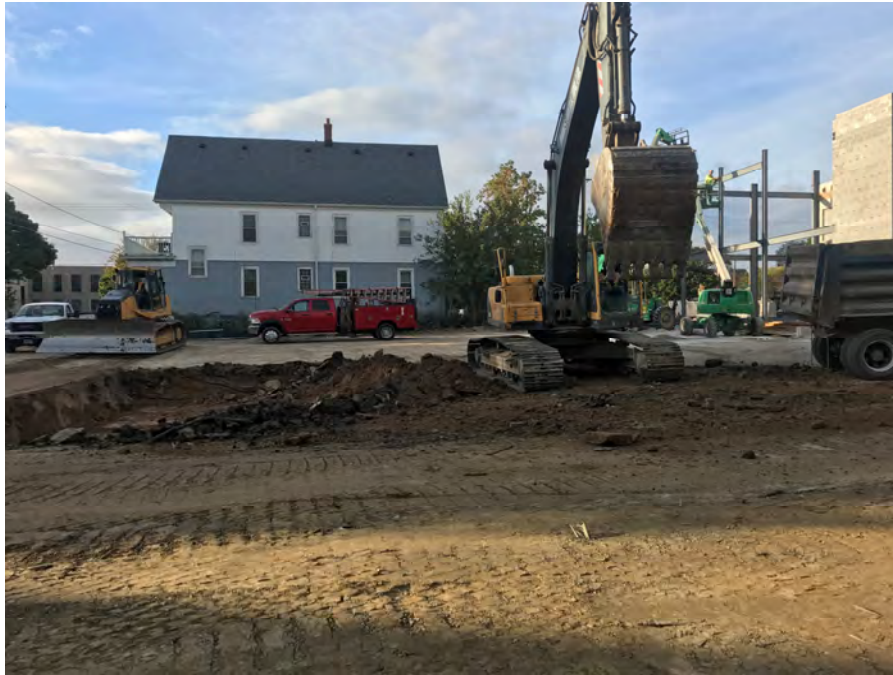
Photo 3: Parking lot subgrade removal (including area for pervious pavers and underlying storm water retention) in progress in northeast portion of Site on October 3, 2017. View looking to south.
