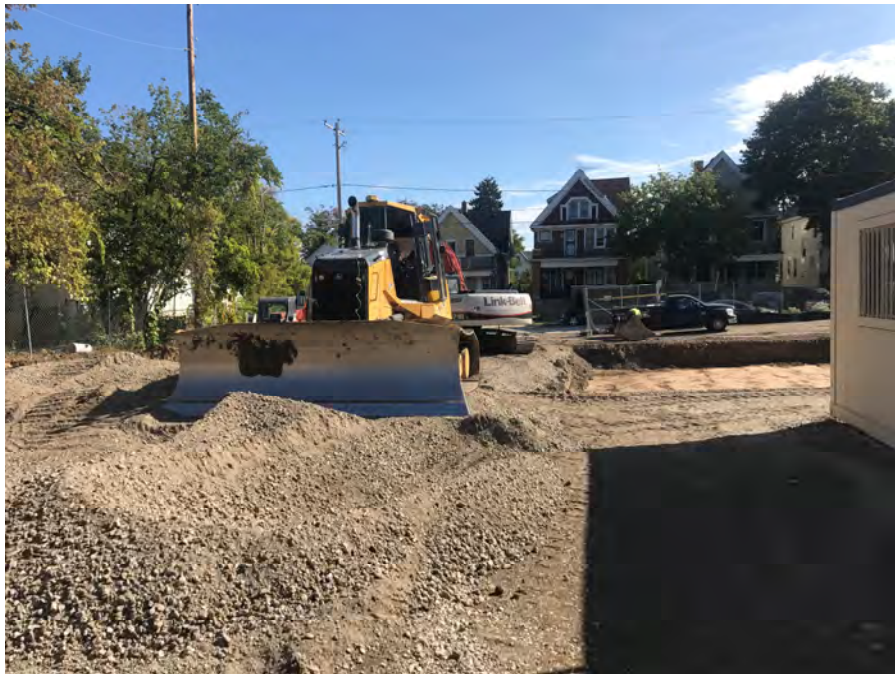
Photo 6: Gravel subgrade being placed in north portion of Site for new asphalt parking lot on October 4, 2017. View looking to east.
