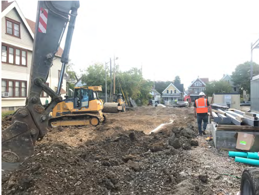
Photo 5: Parking lot subgrade removal in progress in northwest portion of Site on October 4, 2017. View looking to east.
