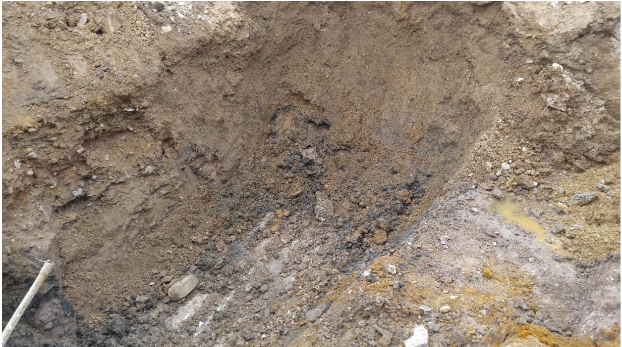
EXCAVATION LIMITS LOOKING EAST SUBSEQUENT TO REMOVAL OF ONE THOUSAND (1,000) GALLON WASTE OIL UST AND OVER- EXCAVATION OF WASTE OIL IMPACTED SOIL
