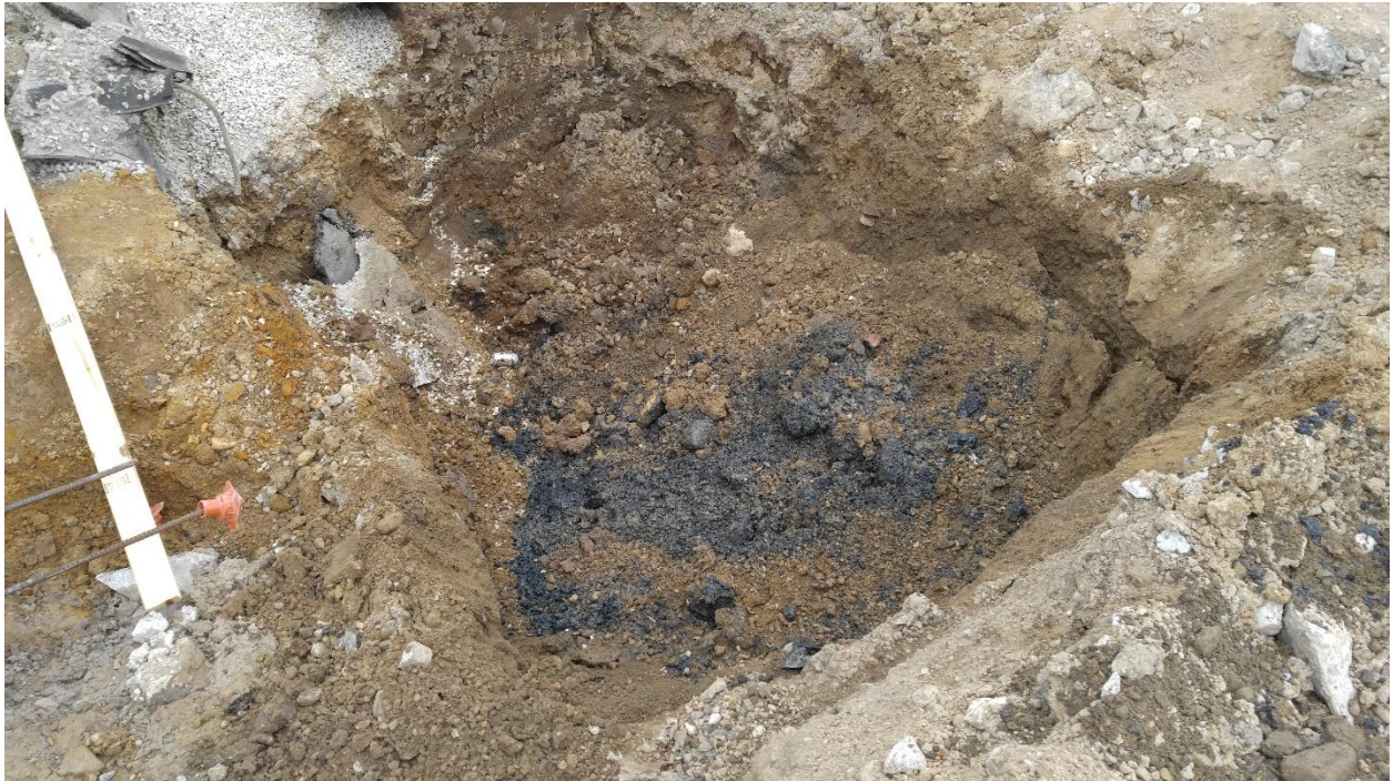
EXCAVATION LIMITS LOOKING SOUTH SUBSEQUENT TO REMOVAL OF ONE THOUSAND (1,000) GALLON WASTE OIL UST
