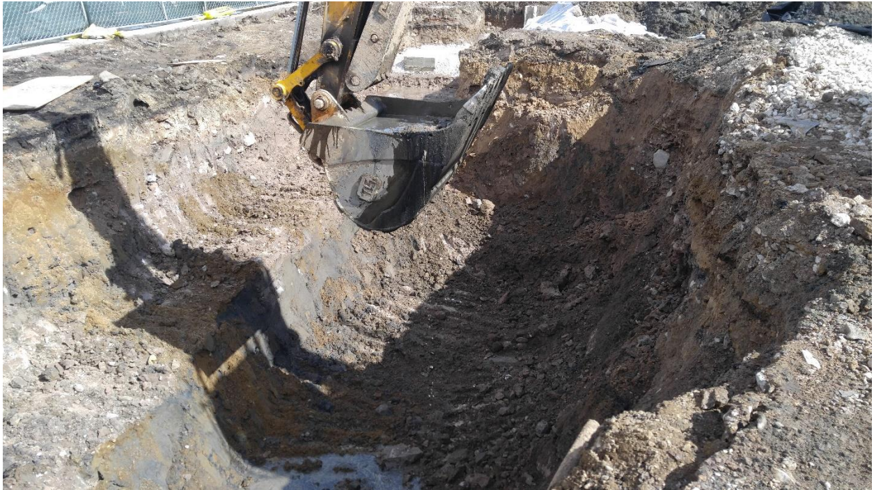
EXCAVATION LIMITS LOOKING EAST SUBSEQUENT TO THE REMOVAL OF THE FOUR THOUSAND (4,000) GALLON UST AND OVER-EXCAVATION OF IMPACTED SOILS
