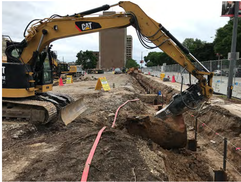
Photo 5: Removal of UST with the help of an excavator. Photo looking north across the site. (Taken 06/22/2018)
