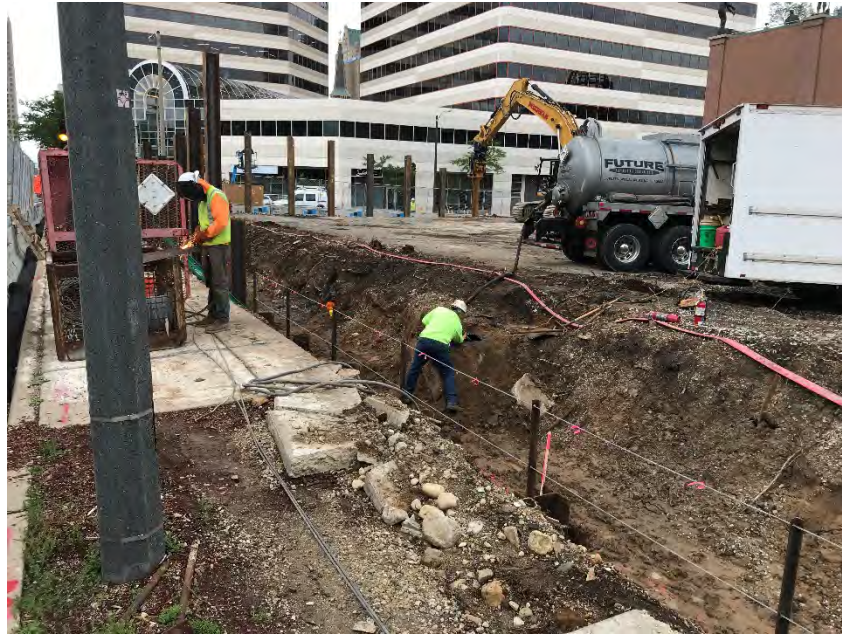
Photo 1: Cleaning and removing 500-gallons of fuel oil and wastewater from UST with Future Environmental vacuum truck. Photo taken along North Milwaukee Street looking southwest across the site. (Taken 06/22/2018)
