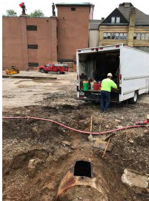
Photo 4: Cleaned UST awaiting removal. Looking west across the site from the east. Grohmann Museum and other MSOE buildings can be seen in the background. (Taken 06/22/2018)
