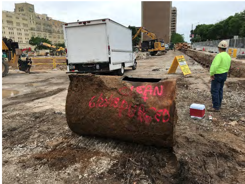
Photo 6: Purged and cleaned tank after removal. Photo looking north across the site. (Taken 06/22/2018)
