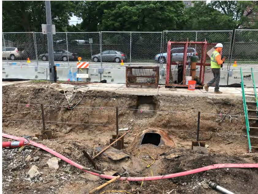
Photo 3: Cleaned UST awaiting removal. Looking east with North Milwaukee Street in background. (Taken 06/22/2018)
