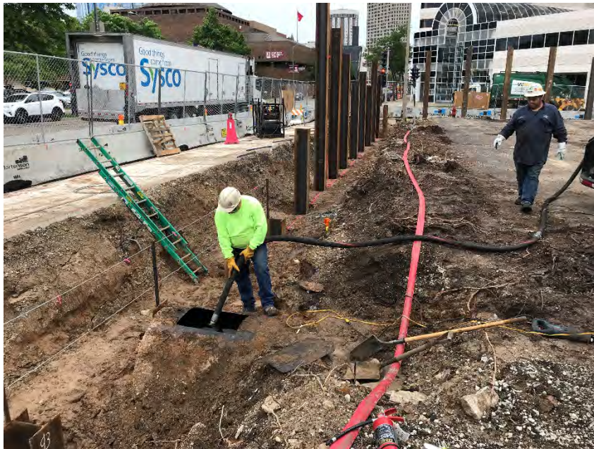
Photo 2: Cleaning and removing 500-gallons of fuel oil and wastewater from UST with Future Environmental vacuum truck. Photo taken looking south across the eastern edge of the site. (Taken 06/22/2018)
