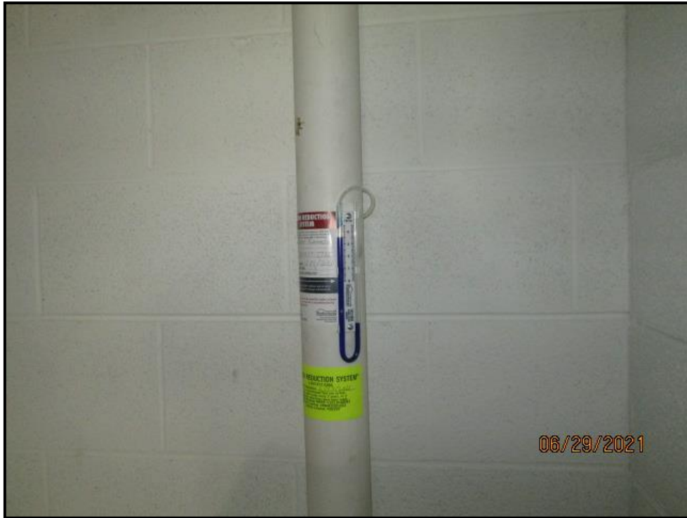
Interior installed manometer on VMS piping (FLC), viewing West.
