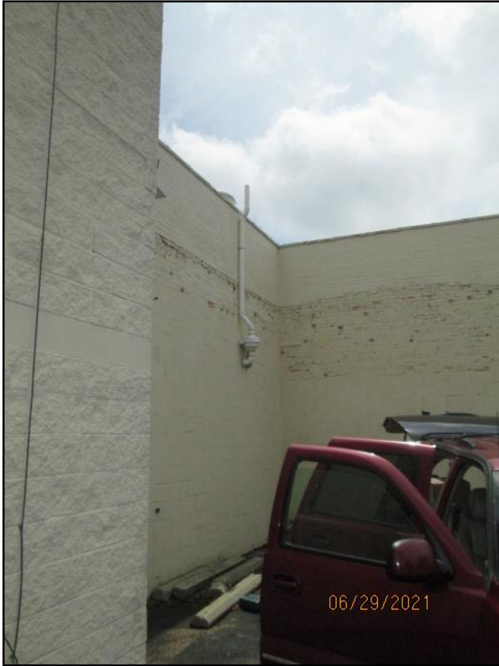
Exterior completed VMS piping with fan (FLC), viewing Southeast.
