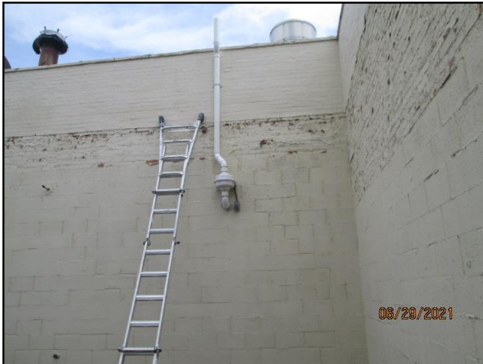
Exterior completed VMS piping with fan and electrical outlet (FLC), viewing East.
