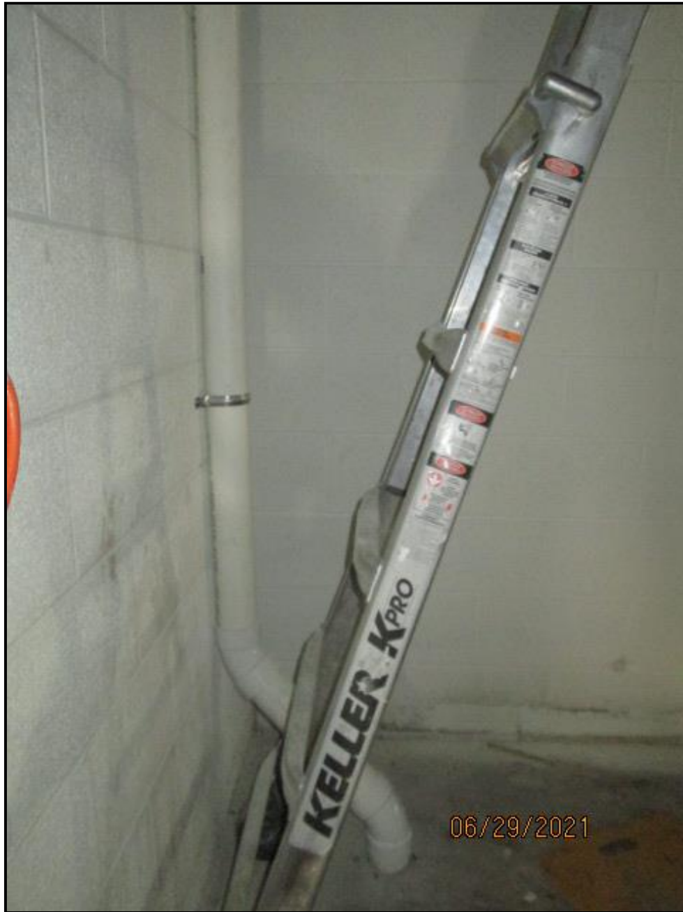
Interior lower piping for Vapor Mitigation System (VMS) (FLC), viewing North.
