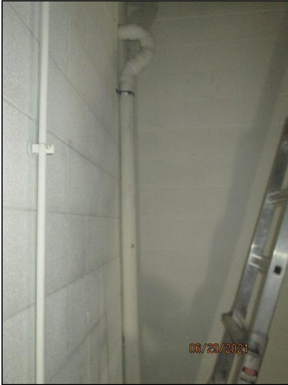
Interior upper piping for VMS (FLC), viewing North.
