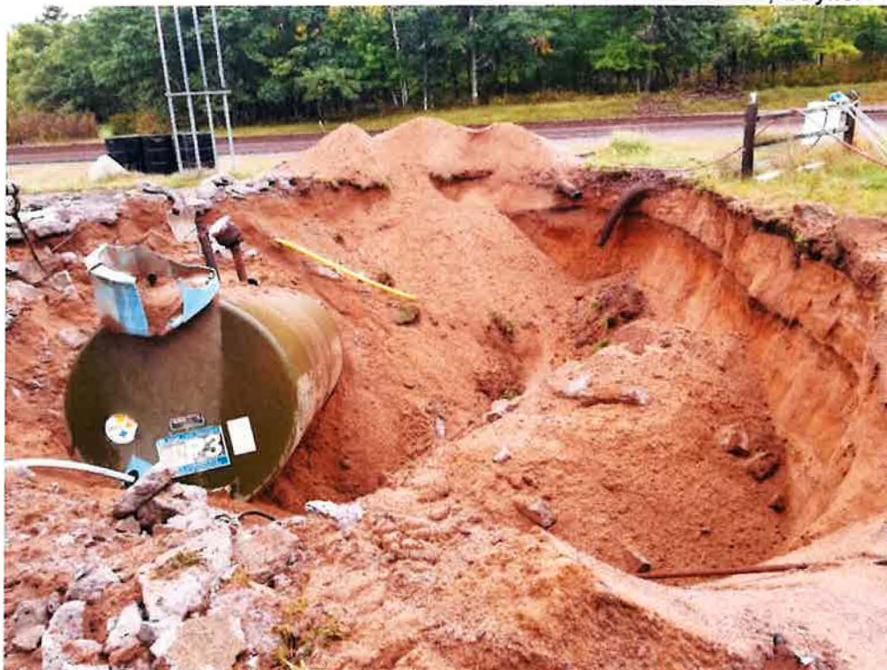
PHOTOGRAPH OF MIDDLE 4,000-GALLON GASOLINE UST
