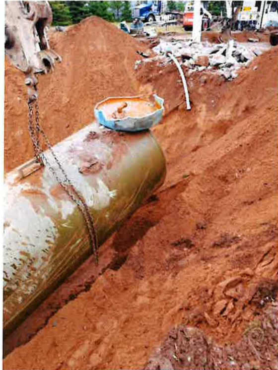
PHOTOGRAPH OF EASTERN 3,000-GALLON UST
