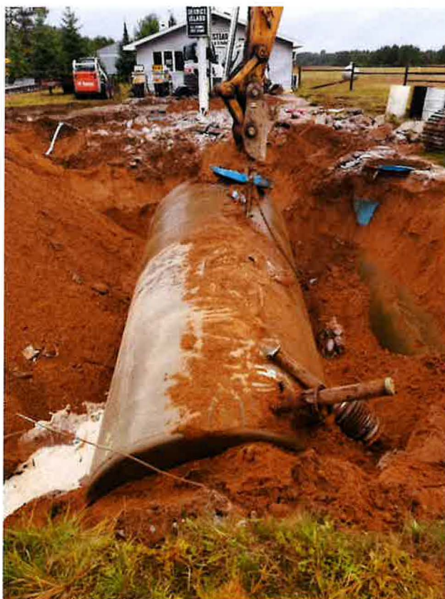
PHOTOGRAPH OF MIDDLE 6,000-GALLON DIESEL UST
