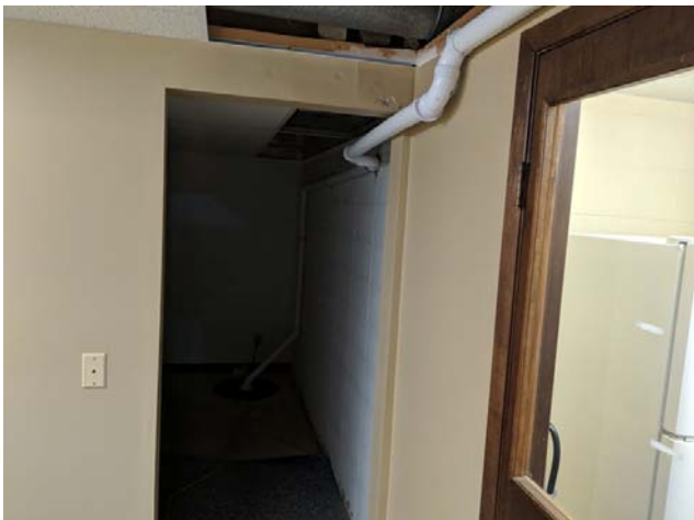
#11: View of southwest pick-up point and associated piping running to the east toward southeast pick-up point.
