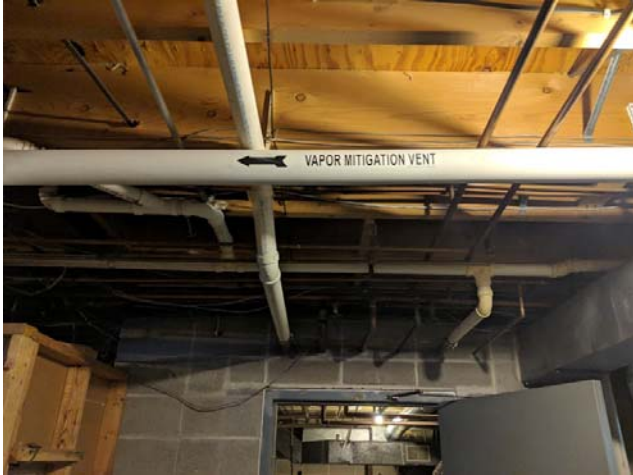
#7: View of VMS piping located on northern portion of basement and labeled.
