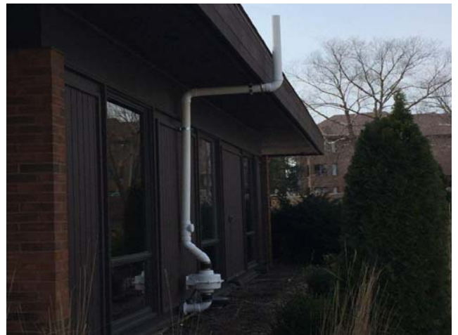
#18: Northern VMS fan and piping on the north side of the building.
