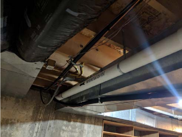
#13: View of southern VMS piping exiting on the south side of the basement.
