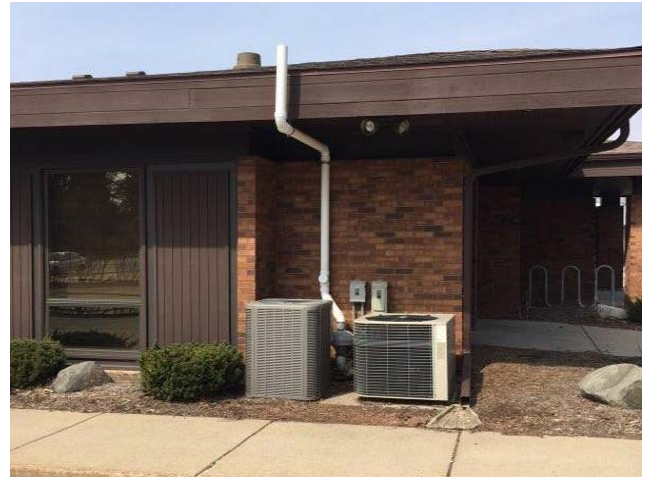
#16: Southern VMS fan and piping on the south side of the building.
