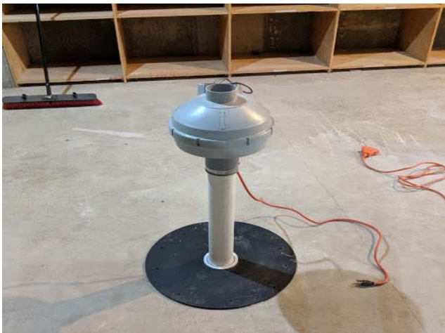
#5: Pick-up point installed and fan temporarily mounted on pick-up point for evaluation of fan requirements.
