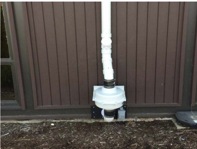
#17: Northern VMS piping exit and fan location.
