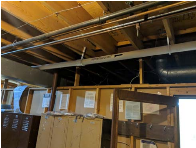
#9: View of VMS piping running along west side of breakroom and labeled.
