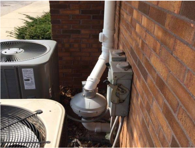
#15: View of exterior southern VMS fan and vent piping.
