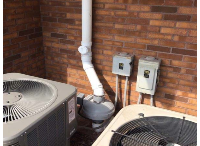
#14: View of exterior southern VMS fan and vent piping.
