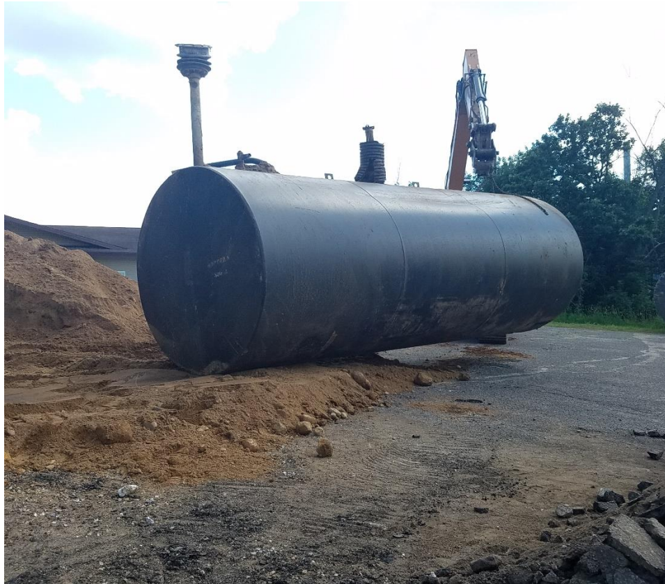
PHOTOGRAPH OF THE 10,000-GALLON GASOLINE TANK
