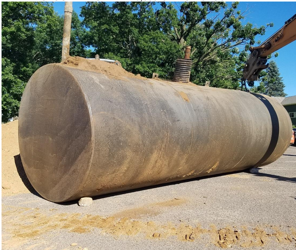
PHOTOGRAPH OF THE NORTH 10,000-GALLON UST
