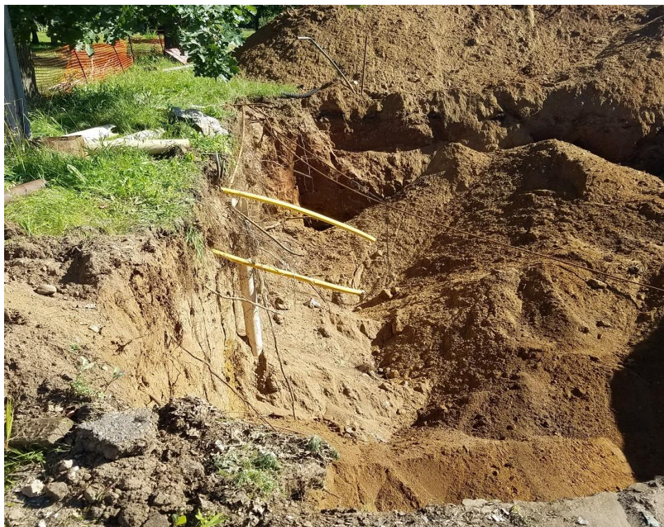
PHOTOGRAPH OF THE FORMER DIPSENER AREA WHICH WERE LOCATED ON THE EASTERN PROPERTY BOUNDARY
