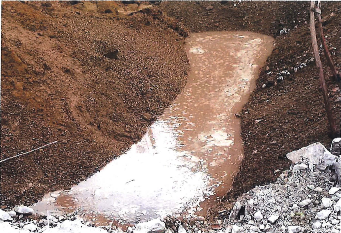
PHOTOGRAPH OF THE WATER BENEATH 8,000-GALLON UST IN THE EXCAVATION
