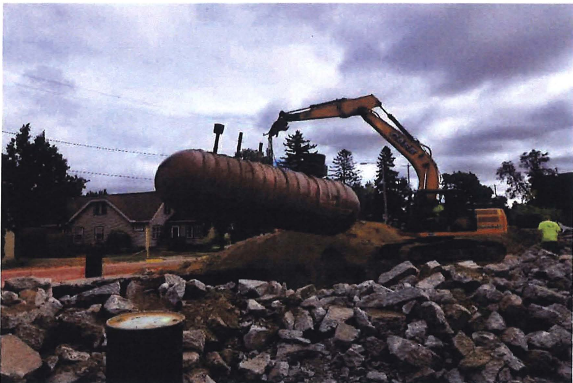
8,000-GALLON UNLEADED GASOLINE UST PHOTOGRAPH OF DISPENSER AREA
