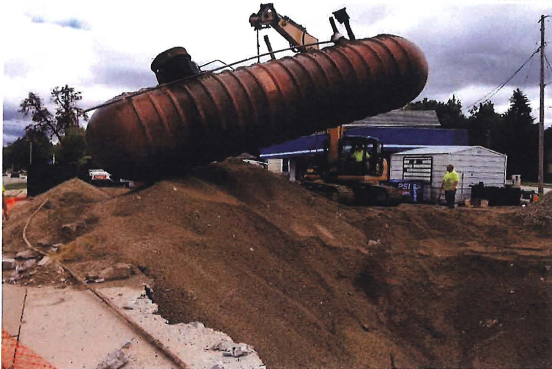
PHOTOGRAPH OF THE 10,000-GALLON UNLEADED GASOLINE UST
