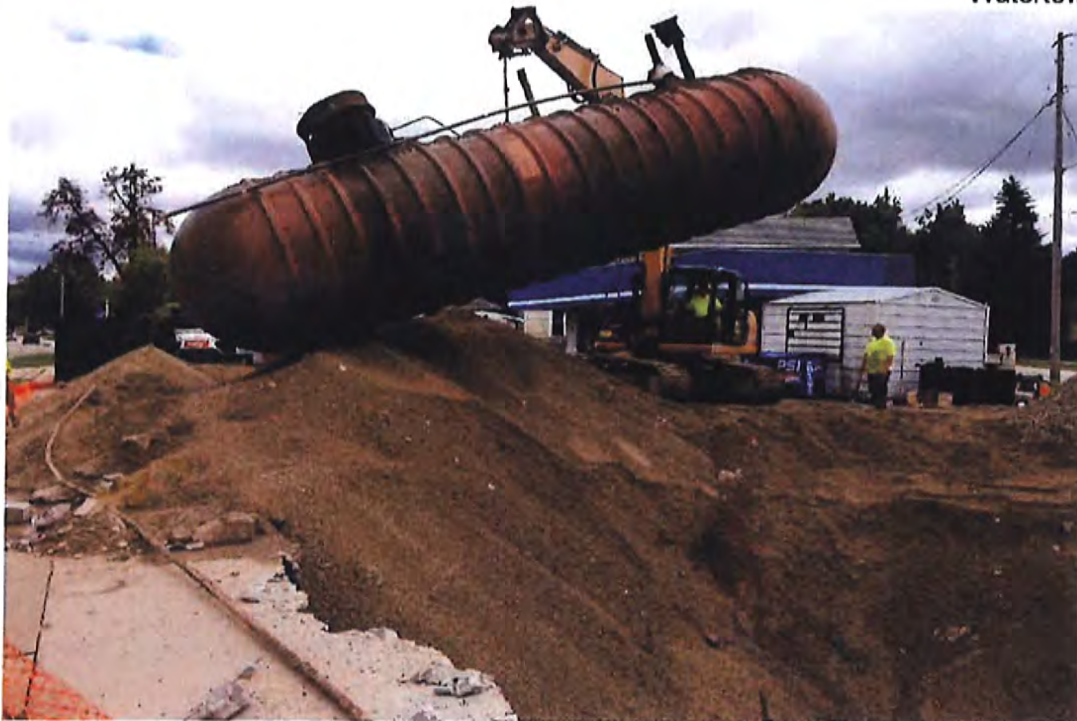
PHOTOGRAPH OF THE 10,000-GALLON UNLEADED GASOLINE UST
