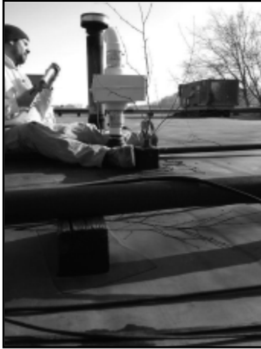
View of the roof-mounted ventilation blower.
