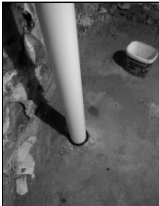
View of the mitigation system piping penetrating the concrete floor slab.
