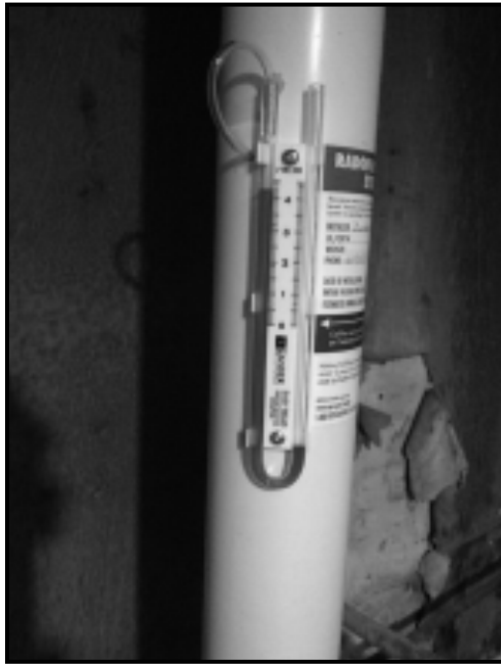
View of the manometer reading 4 inches of water.
