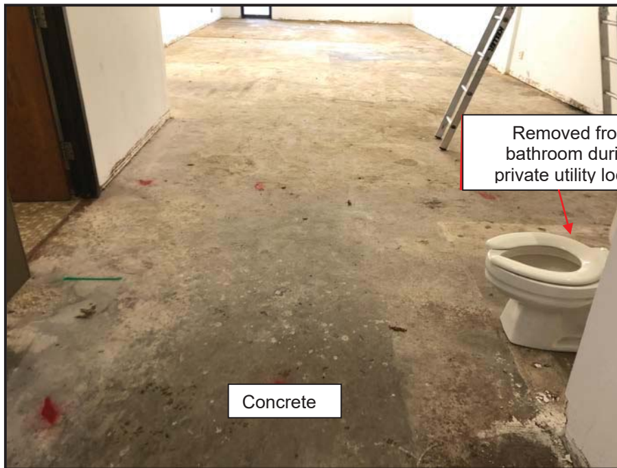
View of the interior of source unit and typical concrete floor to be maintained, facing east.
