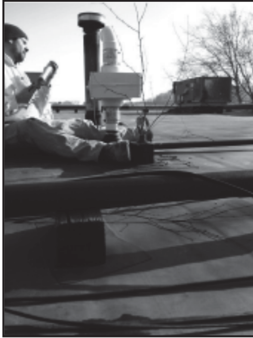
View of the roof-mounted ventilation blower.
