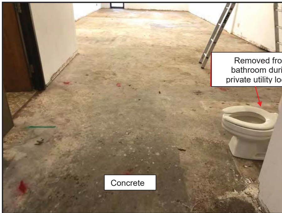
View of the interior of source unit and typical concrete floor to be maintained, facing east.
