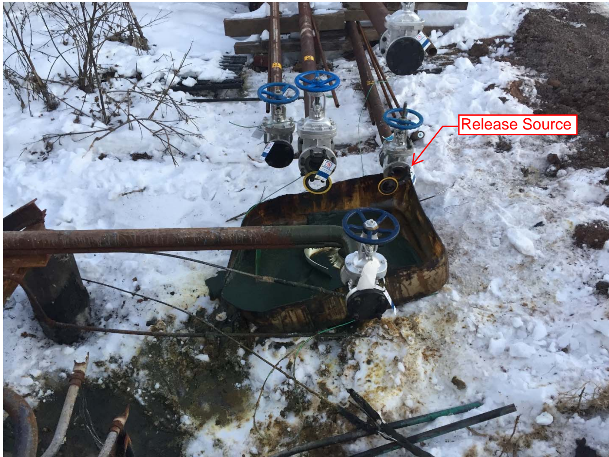
Photo 1: Looking south at the release source and the poly spill containment. #6 fuel oil was meant to slowly drip into the spill containment and be removed with a vacuum truck.
