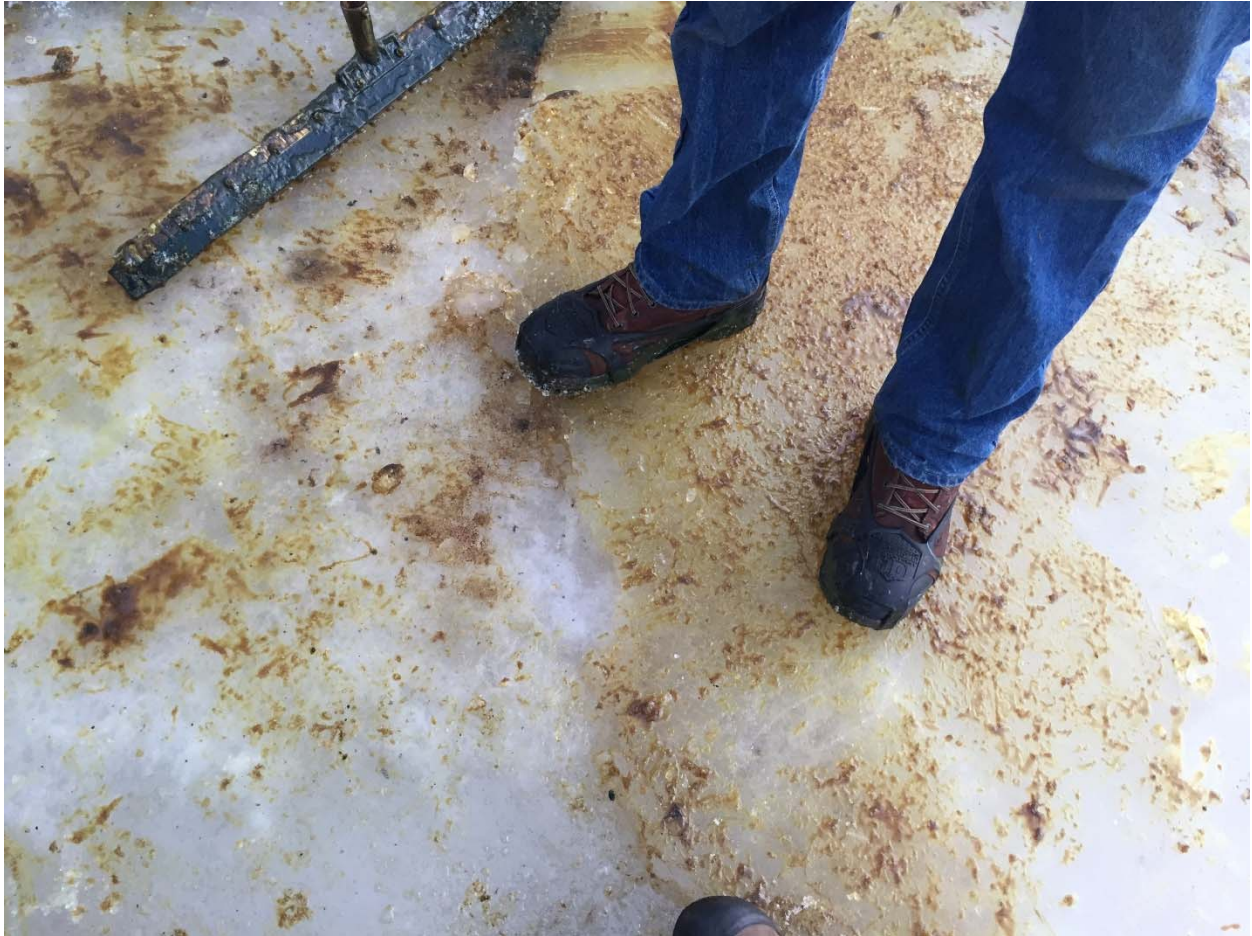
Photo 5: Shovels and squeegees were able to remove the majority of the released #6 fuel oil. The remaining contaminated ice (seen above) was removed with an excavator and shovels before being brought to the contaminated soil storage building.
