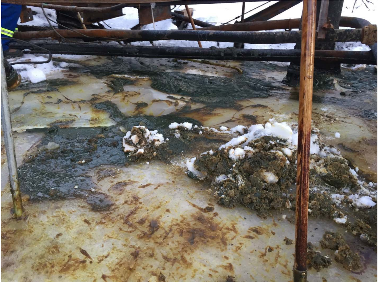
Photo 4: Looking south at the cleanup progression. Piled snow was removed via vacuum trucks. Ice chunks and soil were brought to the contaminated soil storage building.
