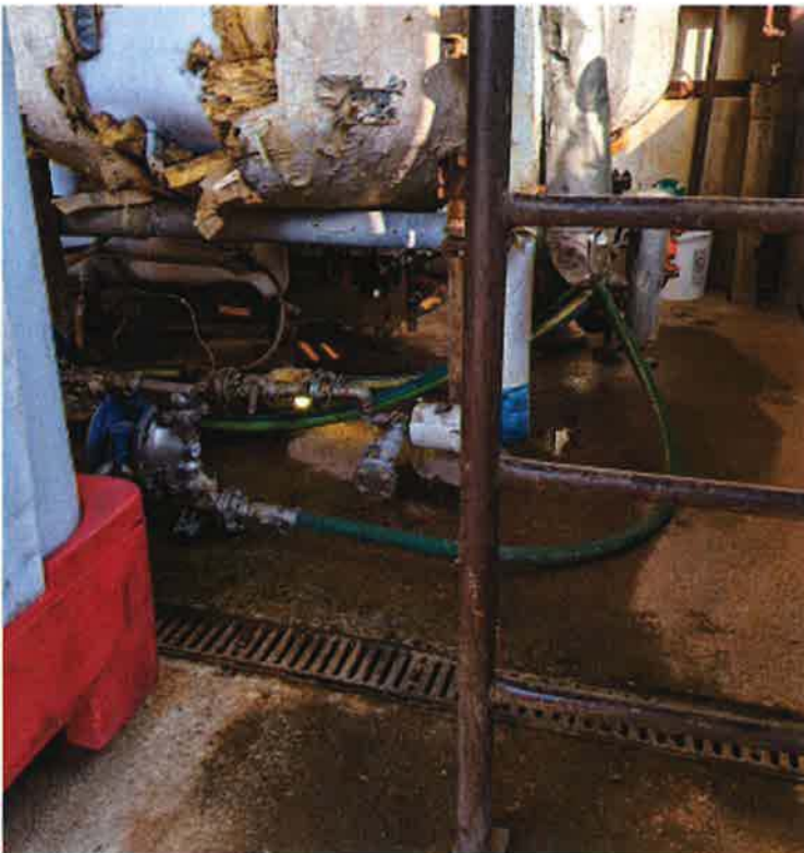
Pic 6 – Base of Vessel 5228, inside 5228's Room
