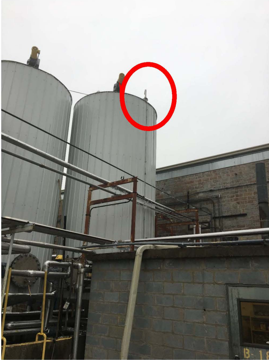
Photo showing vent pipe on blend tank 3.
