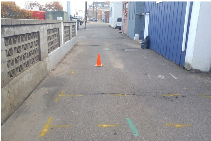
9. Photograph shows the alleyway facing to the east from near the west end and the retaining wall present along the north side of the alley. The highway cone is over SP-9.
