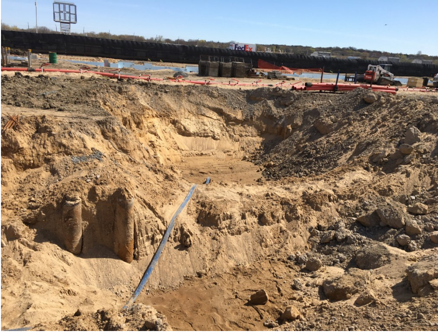
Photo 7: Excavation in loading dock area, looking east - pilings from former building are visible in the left center of photo (4/16/21; 11:06)
