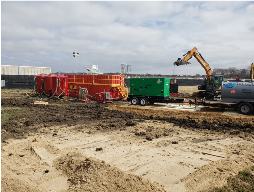
Photo 1: Initial groundwater treatment system setup, looking southeast (3/16/21; 13:21)
