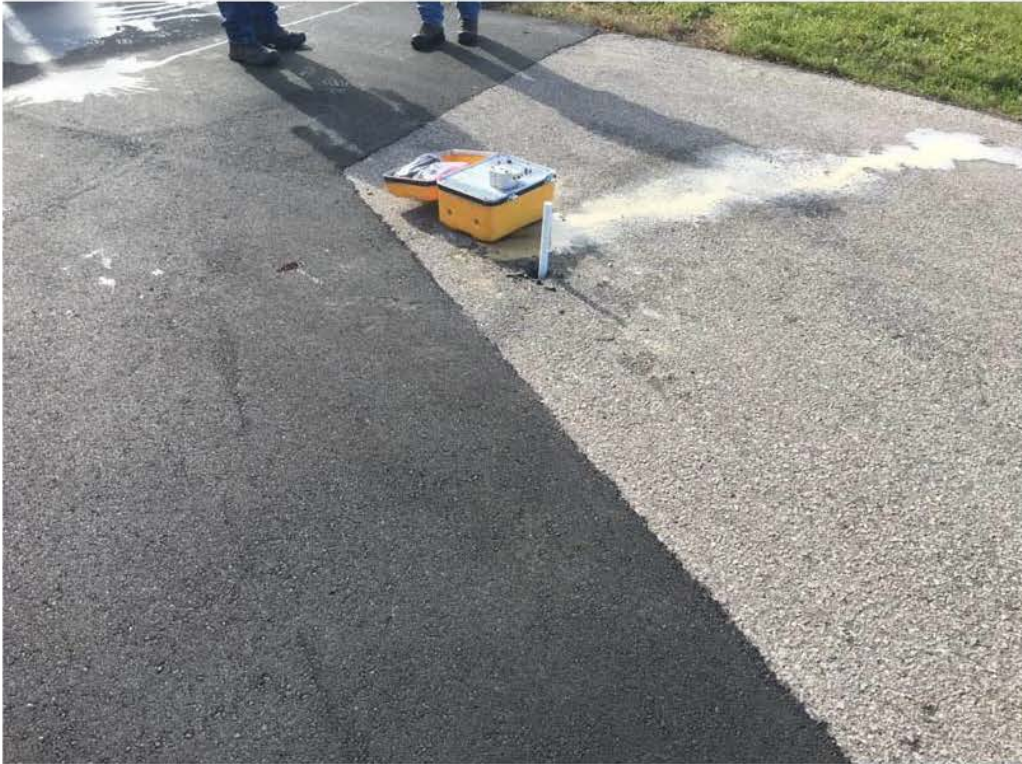
3) Photograph showing temporary monitoring well P-1.
