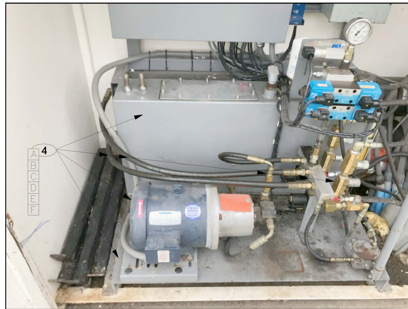
2 BARRIER CONTROL BOX (BCB) MOTOR LINES, RES & VALVES
