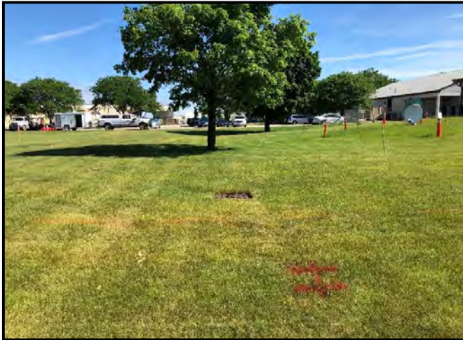
Storm water catch basin.
