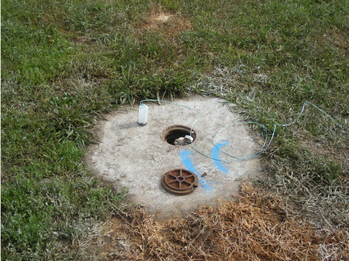
Figure 2 Flush mount monitoring well.
