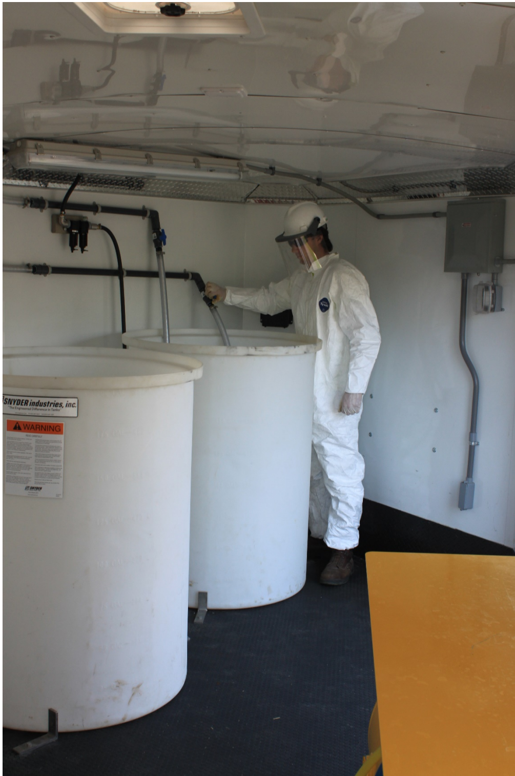
Figure 3 Enclosed chemical mixing system.
