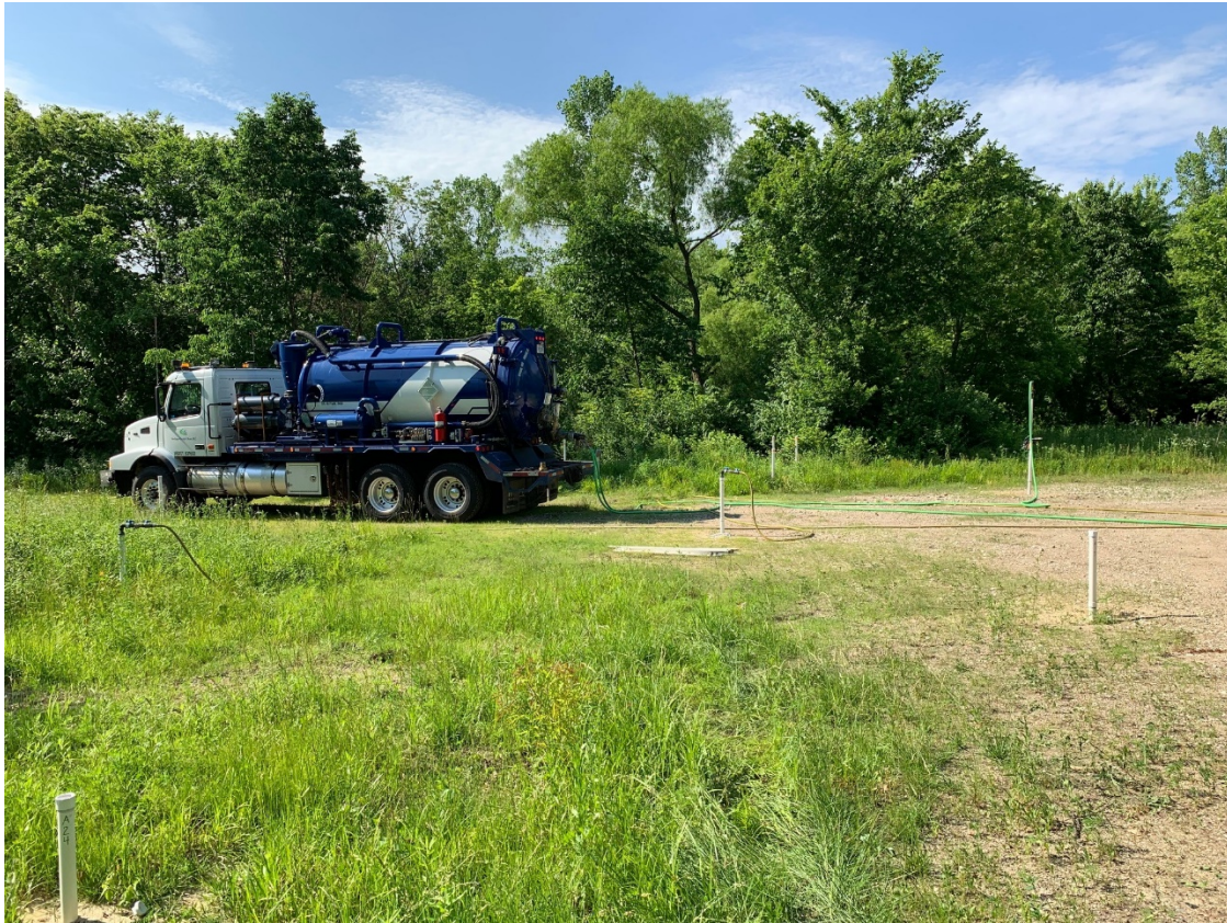
Figure 7 Vacuum extraction truck.
