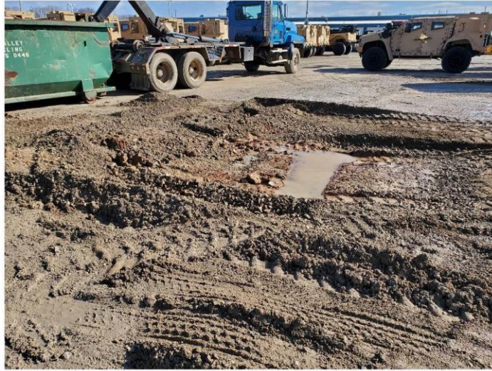
North end of excavation (water is the result of the weeks rain events), view looking east
