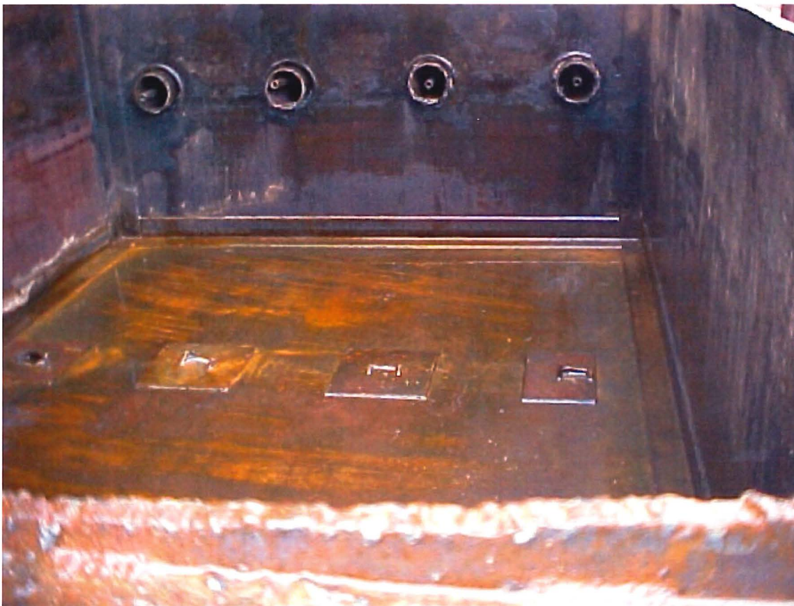
Inside of small evaporator after cleaning.
