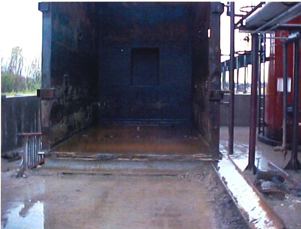
Inside of big evaporator after cleaning.
