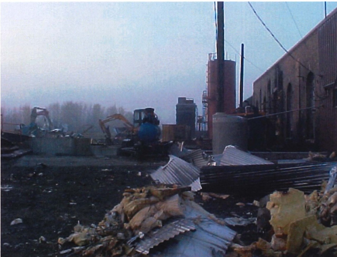
Tank farm on September 29 th after several tanks cleaned and removed for scrap.
