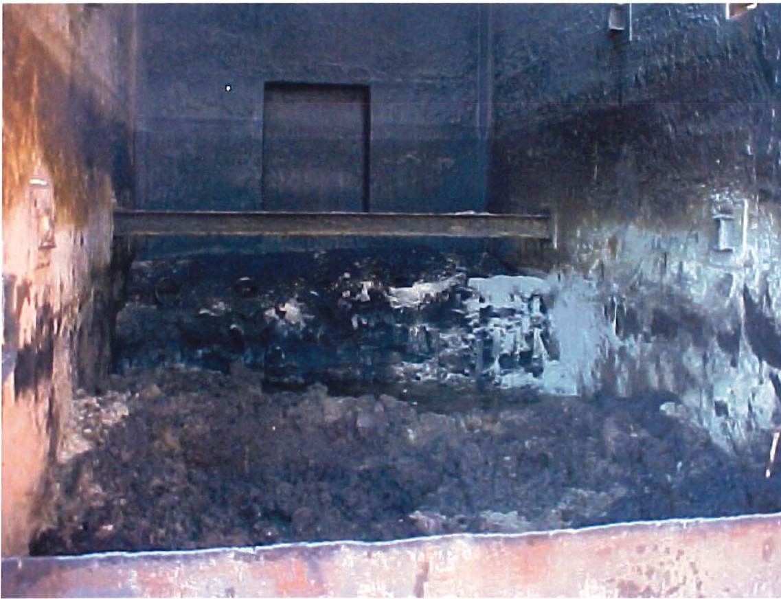
Inside of big evaporator before cleaning.
