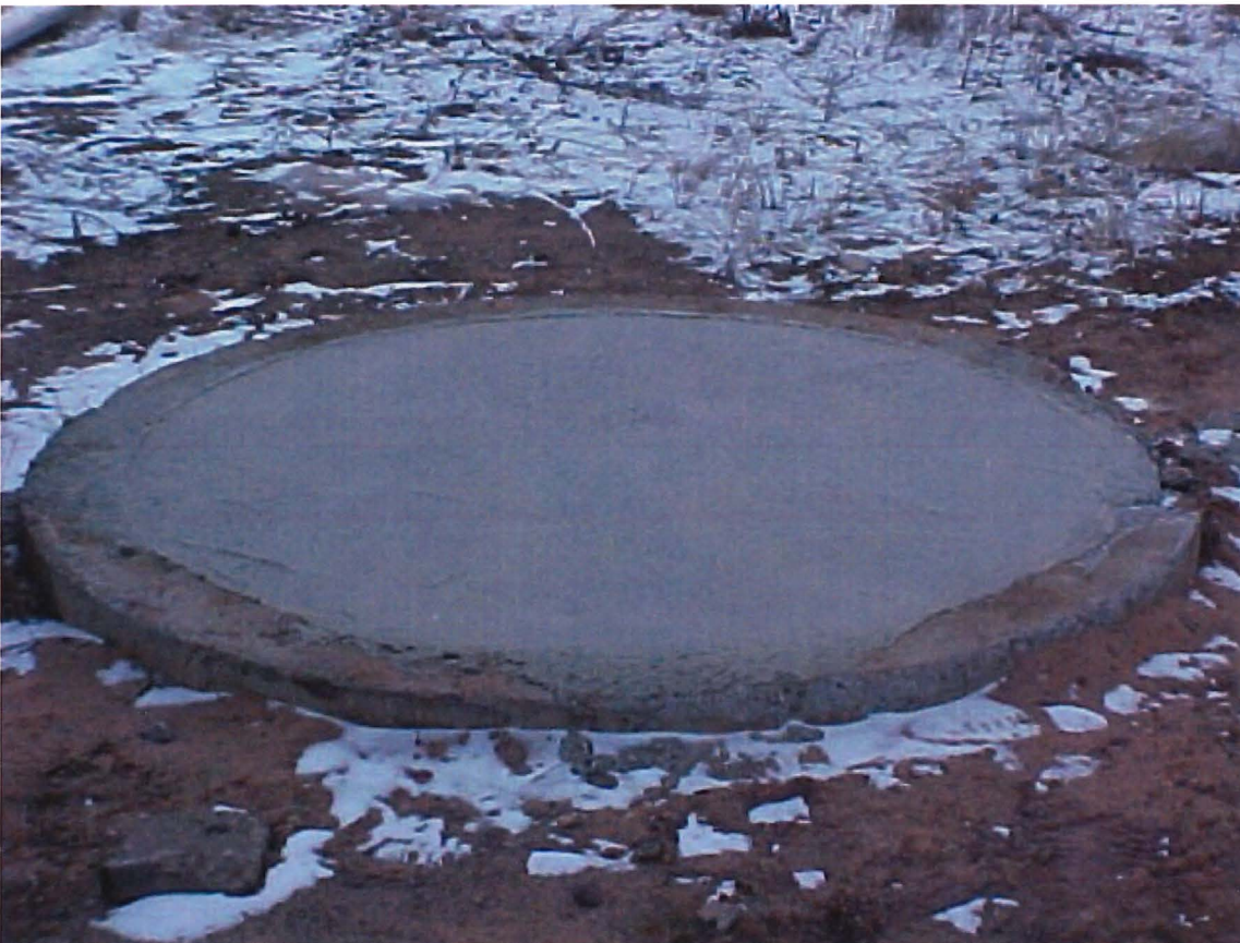
Sumps along drip pad filled with sand and topped with concrete cap to prevent water collection.
