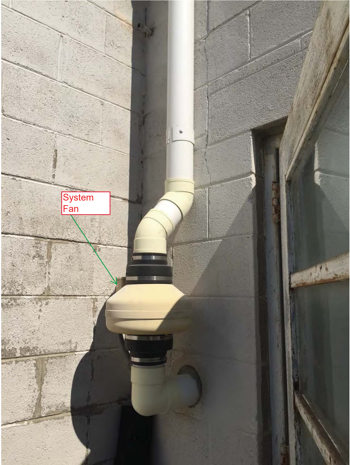
Vapor system located on the west side of the building showing the fan and vent piping going up to the roof line of building.
