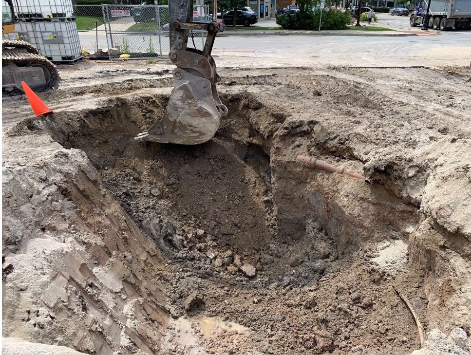
Tank supply pipes inside 8" Clay Tile Lines on west wall of excavation – view South Tanks were approximately at backhoe bucket and further south
