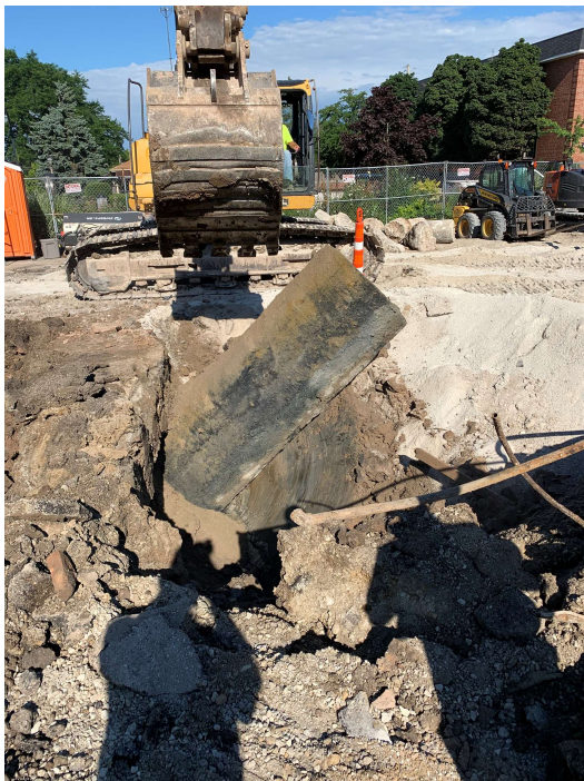
North Tank Removal. South tank still in excavation adjacent Vent pipes run to north
