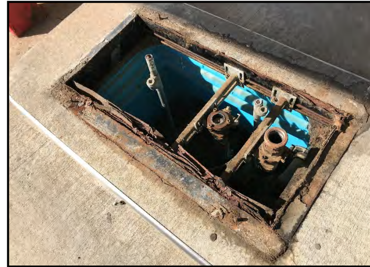
Dispenser sumps beneath gas dispensers
