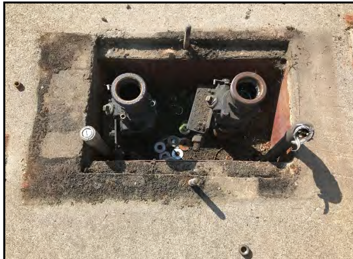
No sumps beneath diesel dispensers
