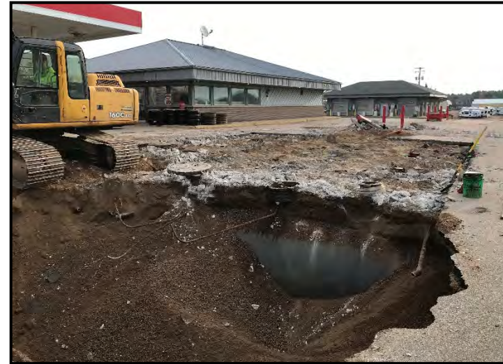
6,000 gallon unleaded UST exposed
