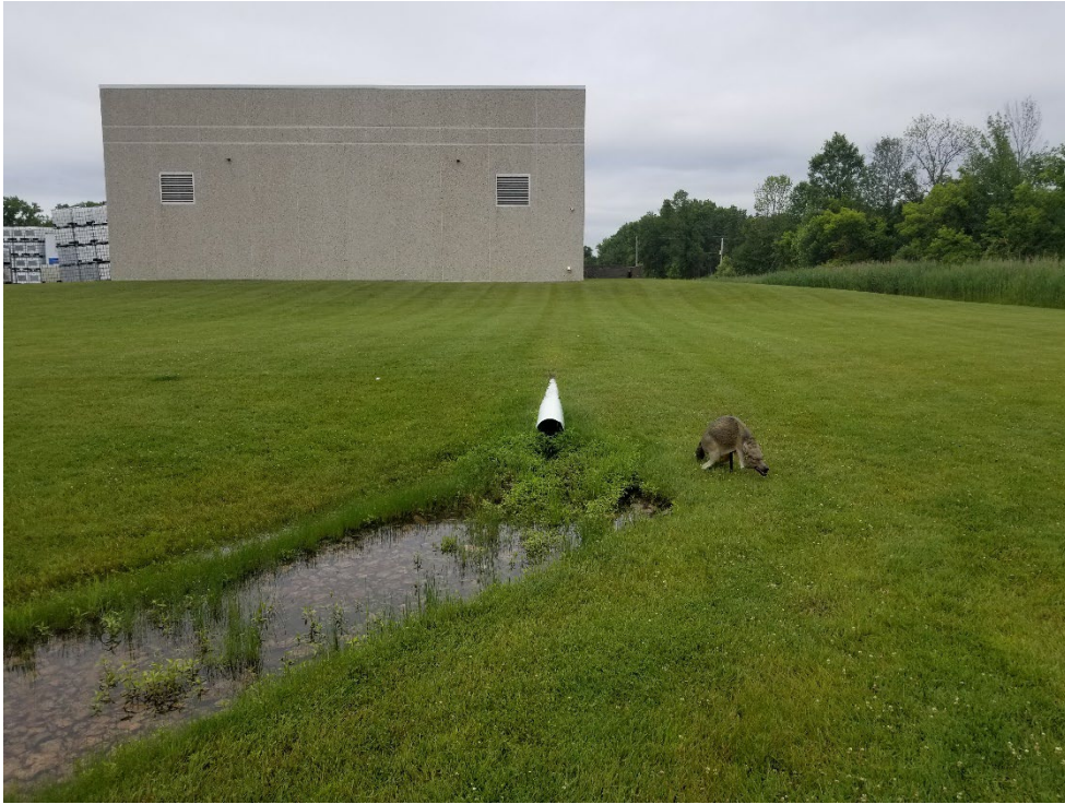
PHOTOGRAPH OF FOUNDATION DRAIN AREA AND SWALE EAST OF OFFICE/PLANT/LAB BUILDING VIEWING WEST
