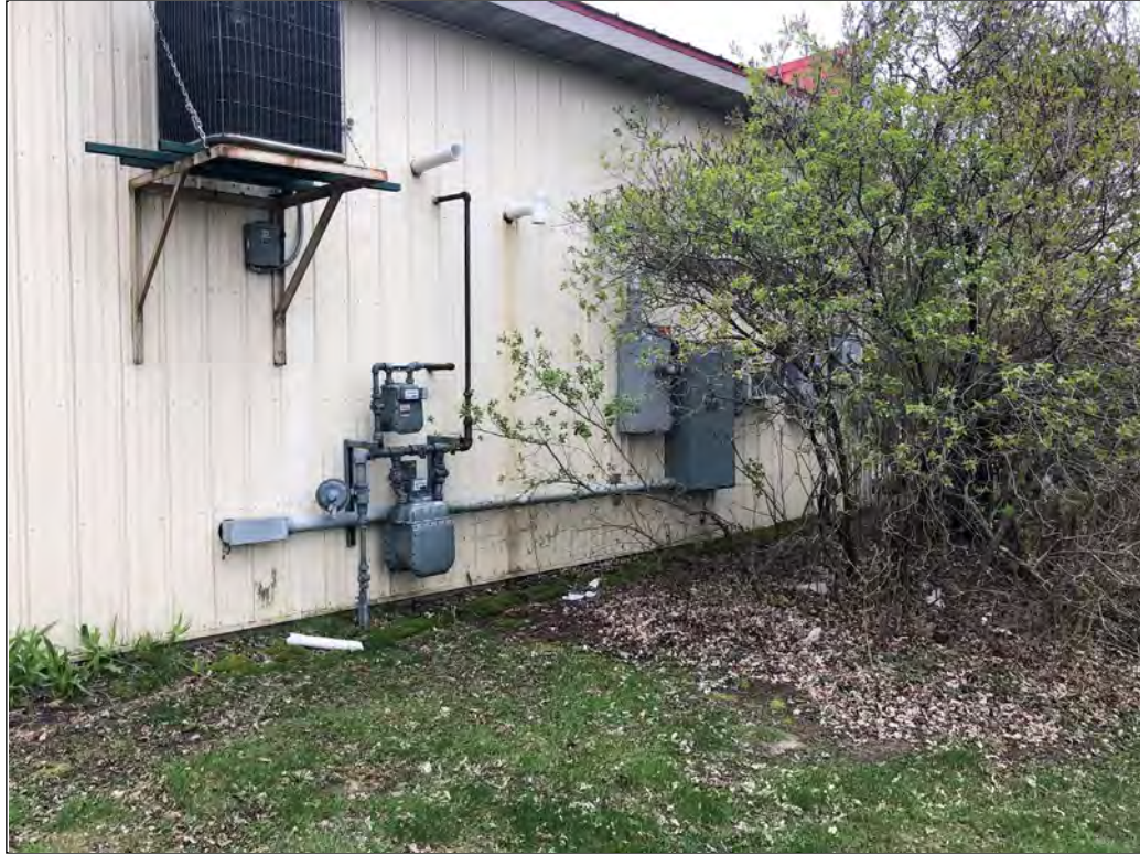
Photo 3: Electrical panels and natural gas meter on the north side of the building.
