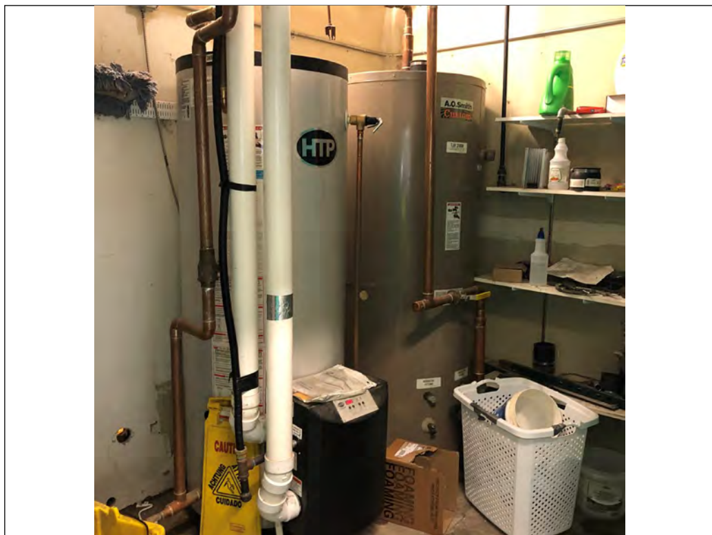
Photo 14: Natural gas water heaters located in storage room.
