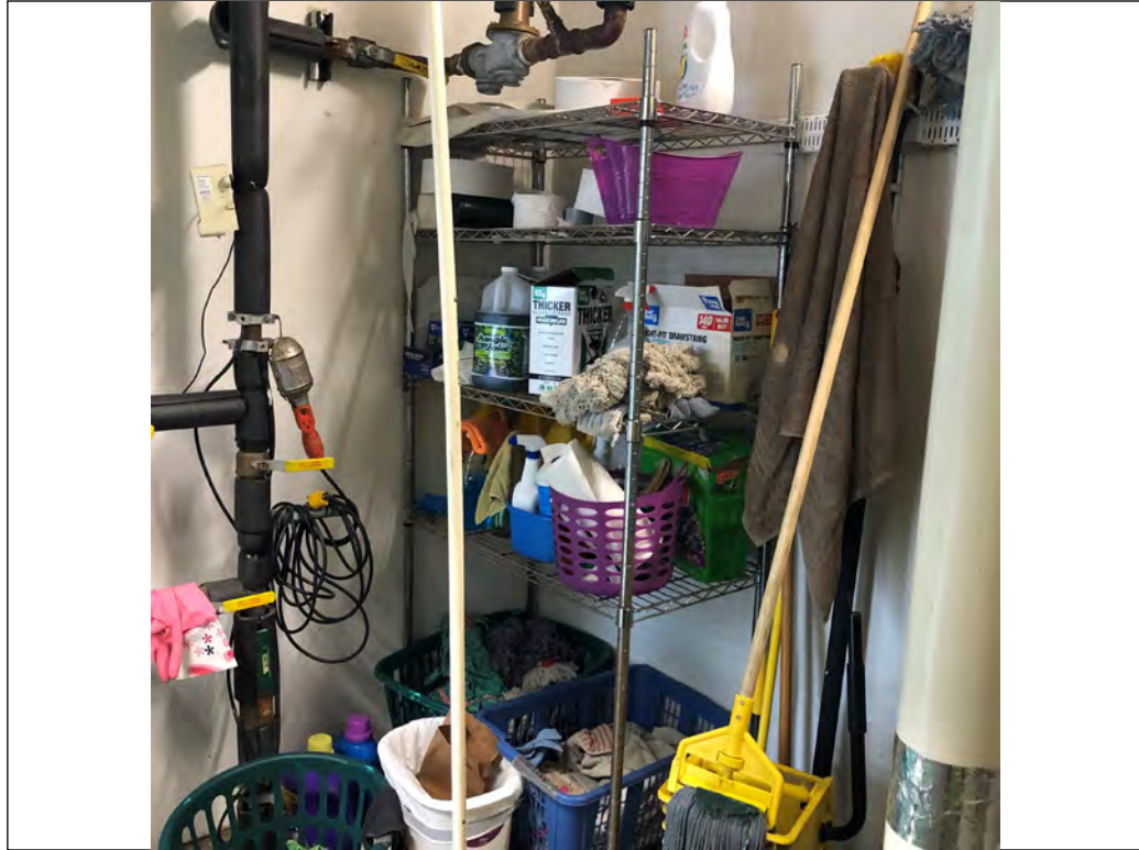
Photo 13: Municipal water line and household cleaning supplies located in storage room.
